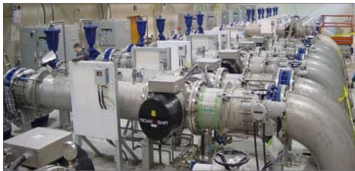
Japan Gulch UV Disinfection Plant
