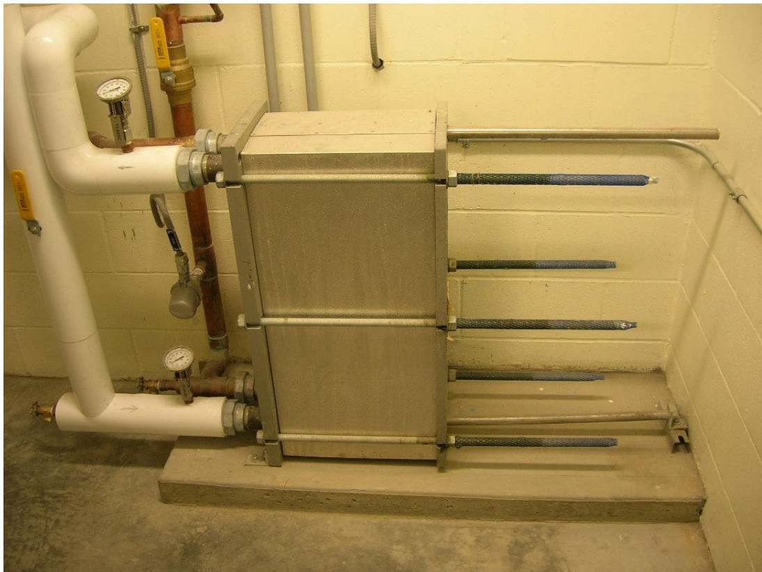
Figure 3 Example of Pumped Plate and Frame Heat Exchanger Installed in a Water Treatment Facility that Uses Lake Water for Heating and Cooling (Source: Associated Engineering)
