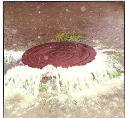
A sewer overflow from a surcharging manhole.
