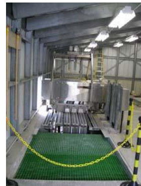
Trojan UV Disinfection
