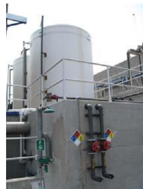
Chemical Delivery Point
