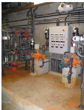
Ferric Chloride Pumps
