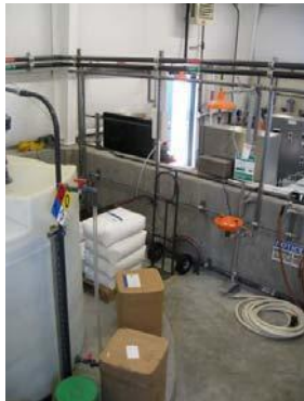
Aluminum Chlorohydrate Tank
