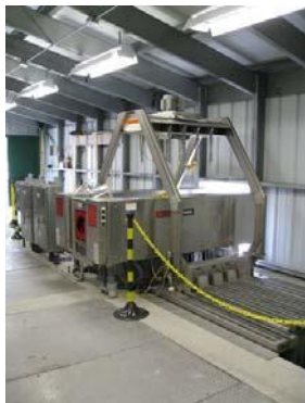
Trojan UV Disinfection
