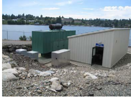
Standby Generator and Electrical Building
