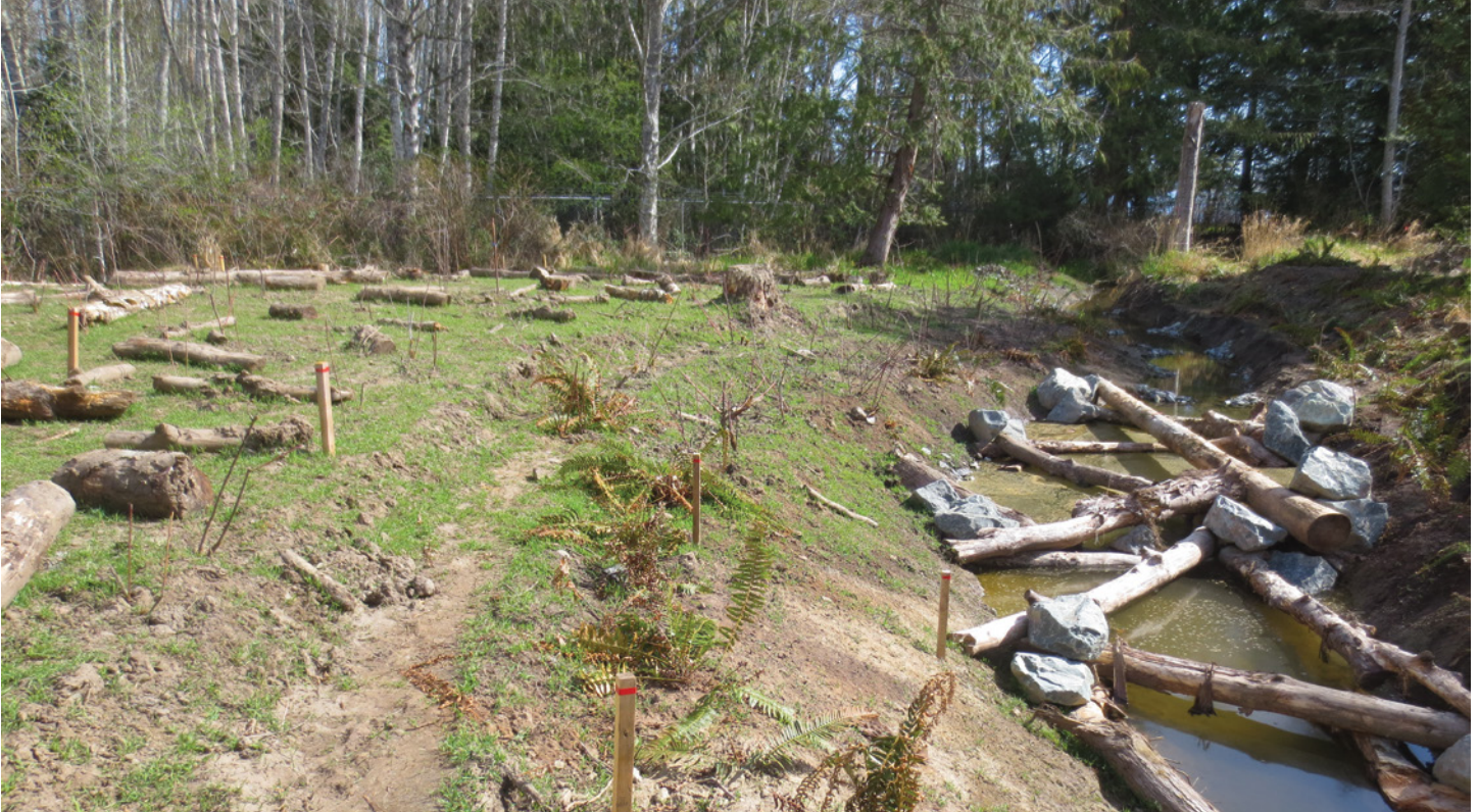
A newly constructed water diversion structure at Pacific Landing is designed to attract spawning fish. Coarse woody debris provides shade and protection from predators, and riparian plants will provide cover and food for insects in the stream.
