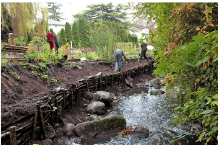
Bioengineering was done to stabilize the creek bank in Oak Bay, though an unusual flood that occurred soon after meant that the work needed to be redone. PHOTO CREDIT: Matthew Wheeler
