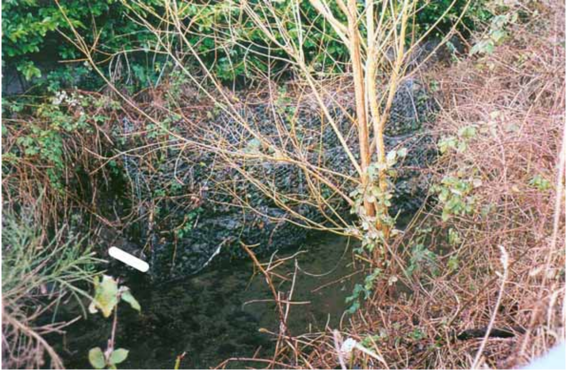
PLATE 11. Zone 6 of Bowker Creek showing gabion wall on west bank downstream of foot bridge with planted laurel hedge on top of bank.
