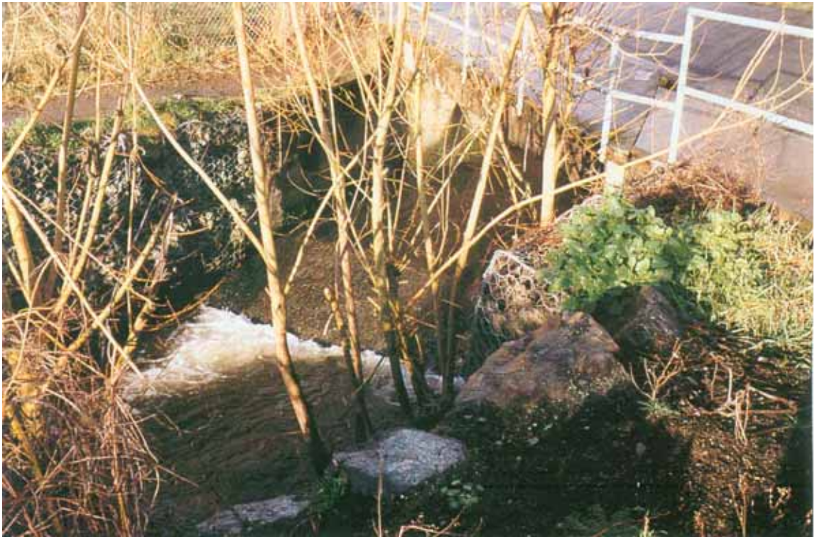
PLATE 6. East bank of Bowker Creek in Zone 3 showing golden willow growth along gabion wall at the outlet of the Haultain Road culvert.
