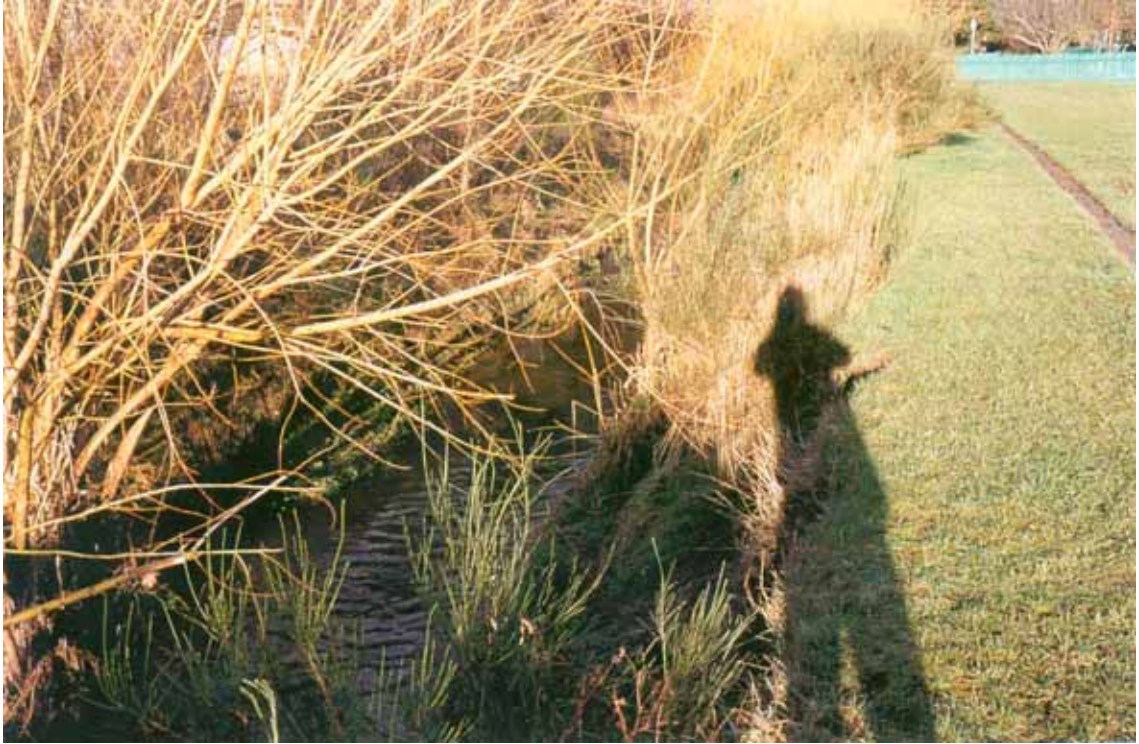
PLATE 3. Zone 2 of Bowker Creek adjacent to Royal Jubilee Hospital showing eroding east bank and existing riparian vegetation community.
