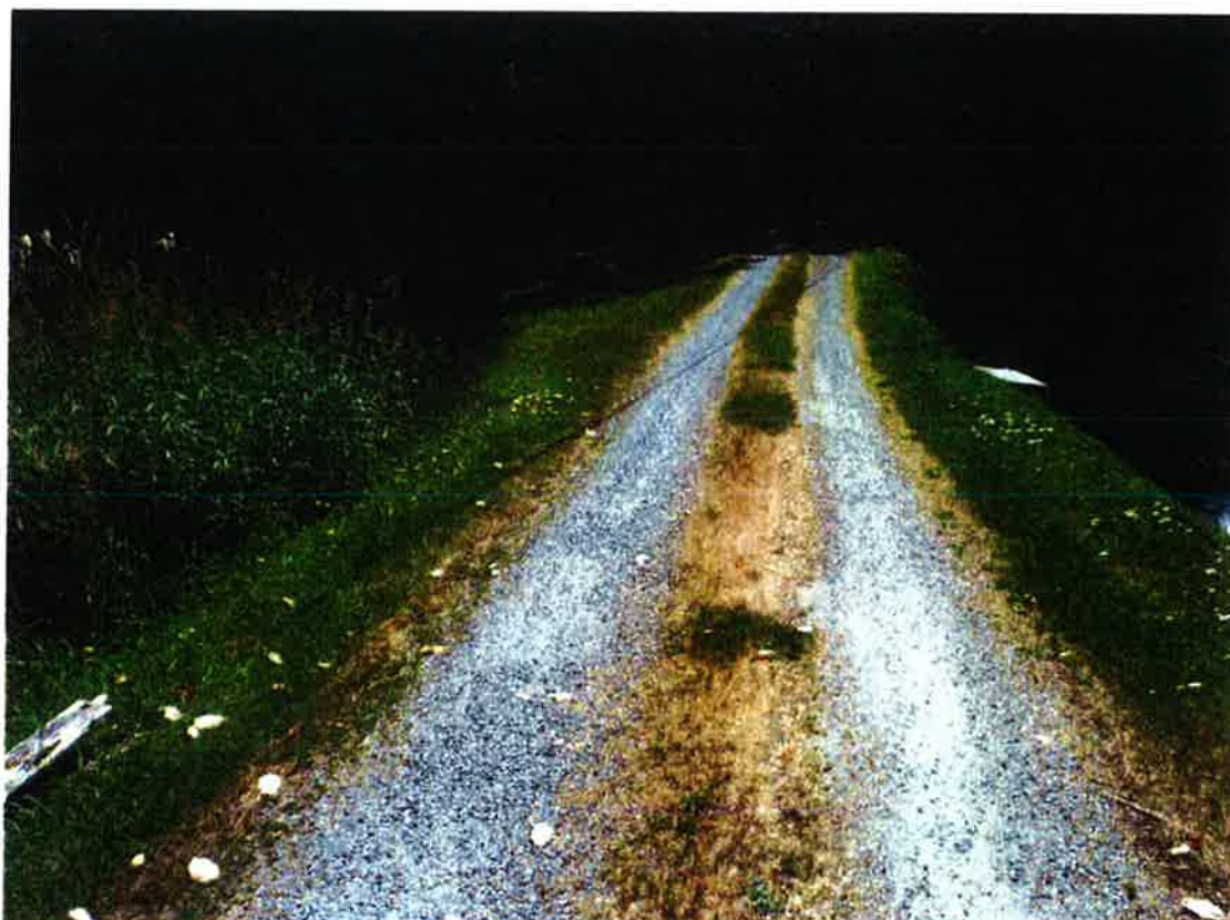
Gardom Pond Dam – Ruts in the road on the dam crest should be filled. Upstream face should be brushed to facilitate inspection.
