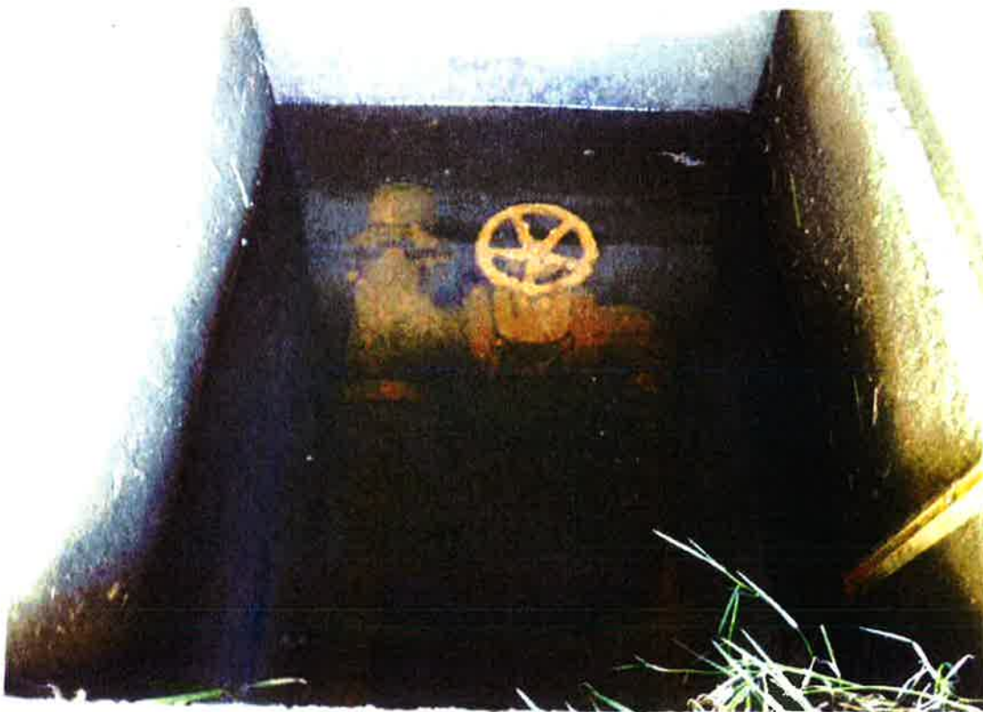
Gardom Pond Dam – Valve chamber at downstream. Drain pipe should be installed to keep chamber dry and to monitor seepage into the chamber.
