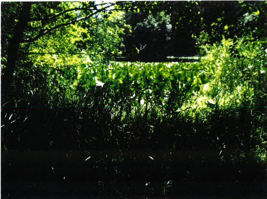
Gardom Pond Spillway Outlet – Remove vegetation leading up to channel.
