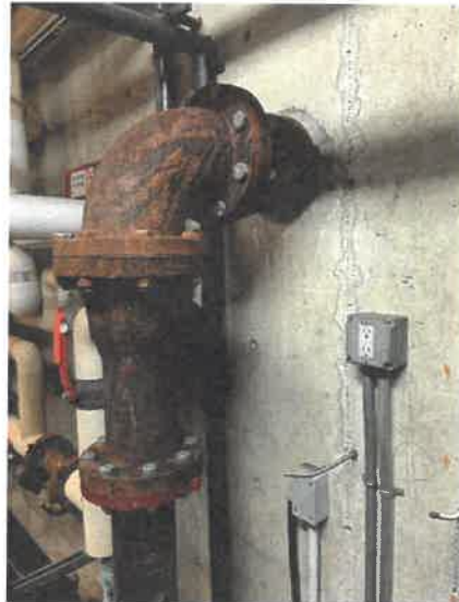
Exposed Domestic Water Piping Corroded
