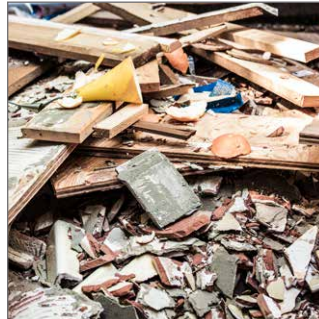
CLEAN DEMOLITION WASTE (commercial)
