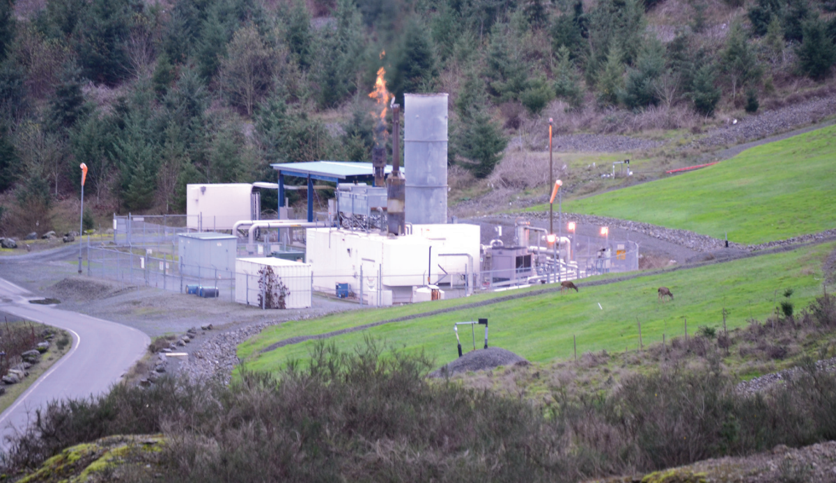
Hartland Gas Utilization Facility
