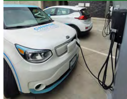
Fleet EV charging at McLoughlin Point Wastewater Treatment Plant
