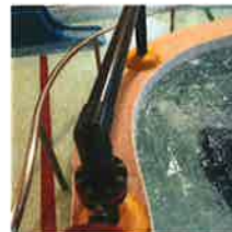
STEEL POOL SPRAY FEATURES REPLACED WITH PVC
