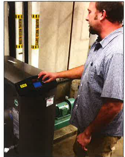
SEAPARC Administrative Coordinator Nathan Stewart studies the display screen on the new boiler.
