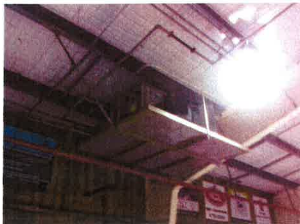
Fig. 2 – Munters Dehumidifier installed in 2009
