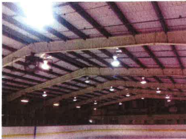
Fig. 3 – Corrosion on Arena Structure Facing Away from Lobby
