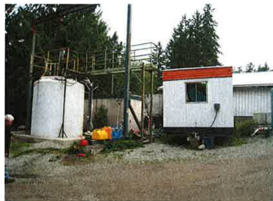
Membrane Bio Reactor tank and operator facilities.
