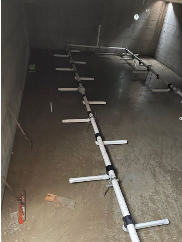
Diffusers installed in WWTP Tank
