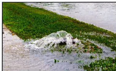
Overflowing sewer manhole.
