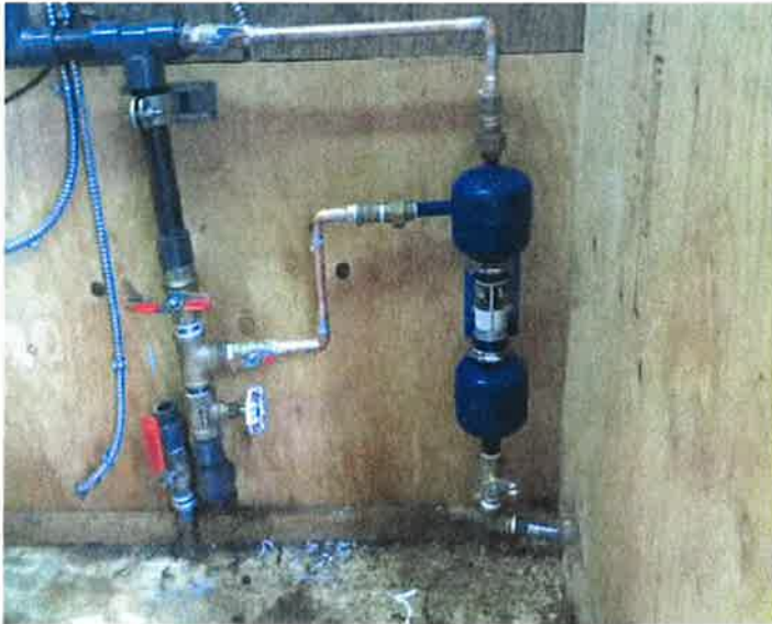
Figure 1. Vortex Filter Installed in Pumphouse
