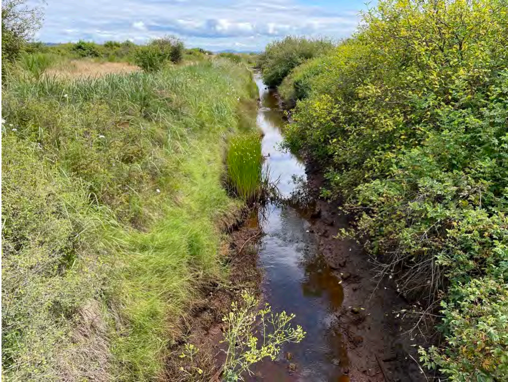
Lamont ROW looking east toward the tide gate July 16, 2022. Water was actively flowing toward the trash rack (seaward).
