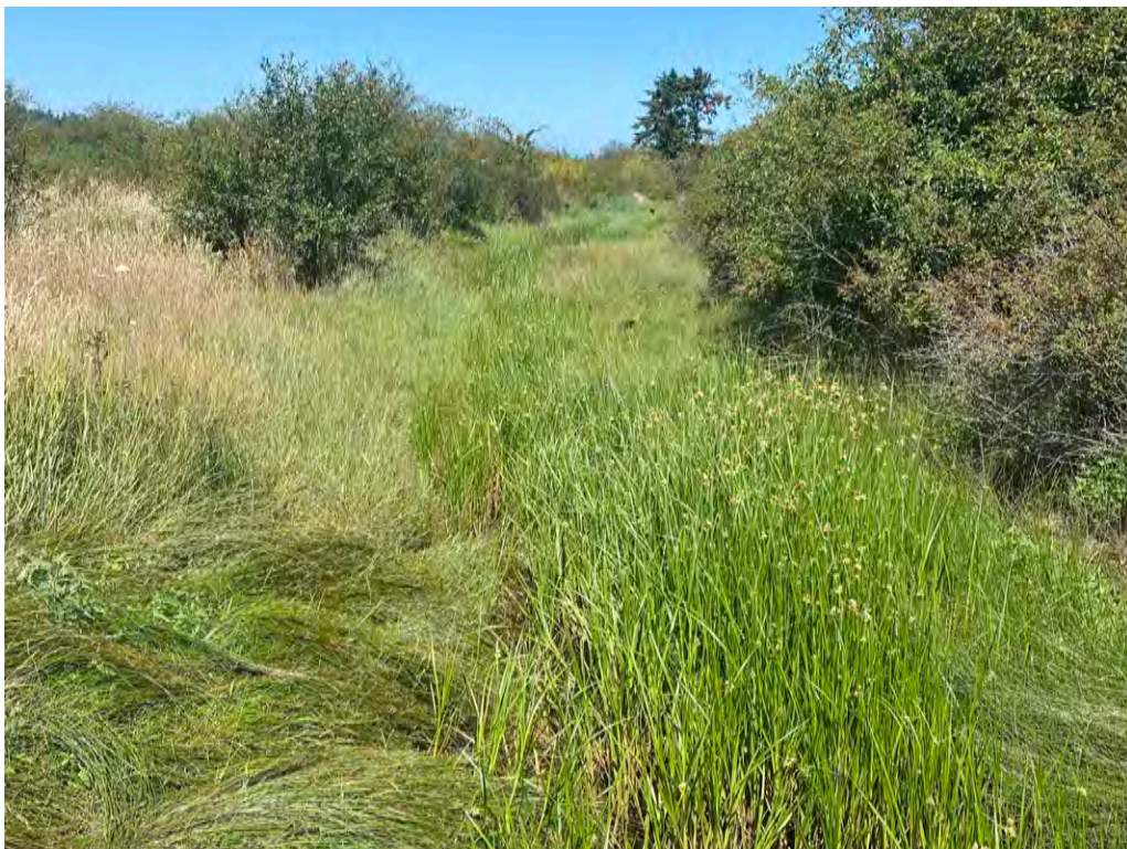
Campground ditch looking north July 5, 2021 prior to 2021 maintenance.
