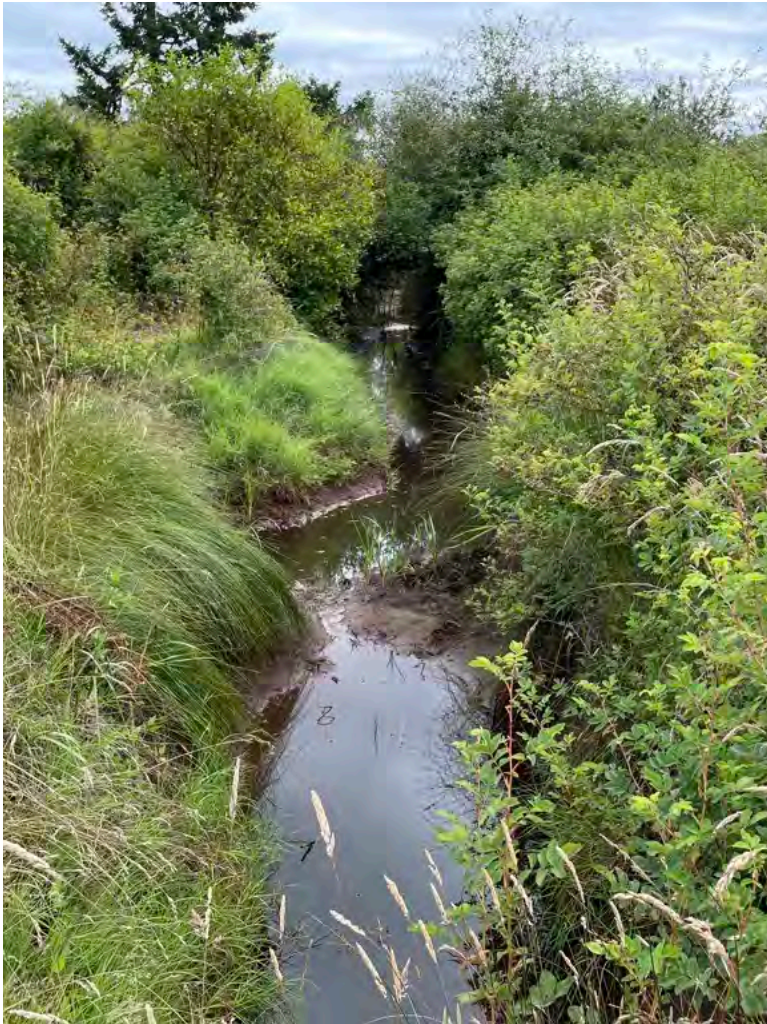
Confluence of Lamont Road ROW and Ditch 4 July 16, 2022. Note the clear open channel as a result of last year's maintenance.
