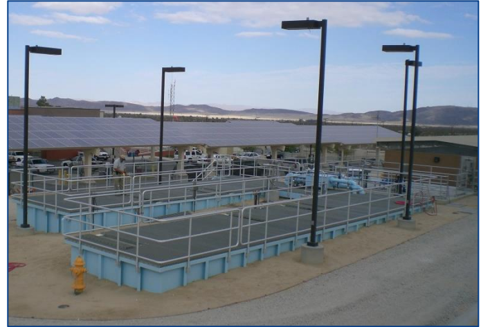
Joshua Basin WWTP, California
