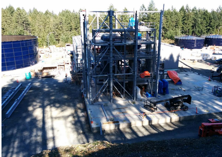
Figure 8- Residuals Treatment Facility- Installation of structural steel for Dryer Building exterior frame ongoing.
