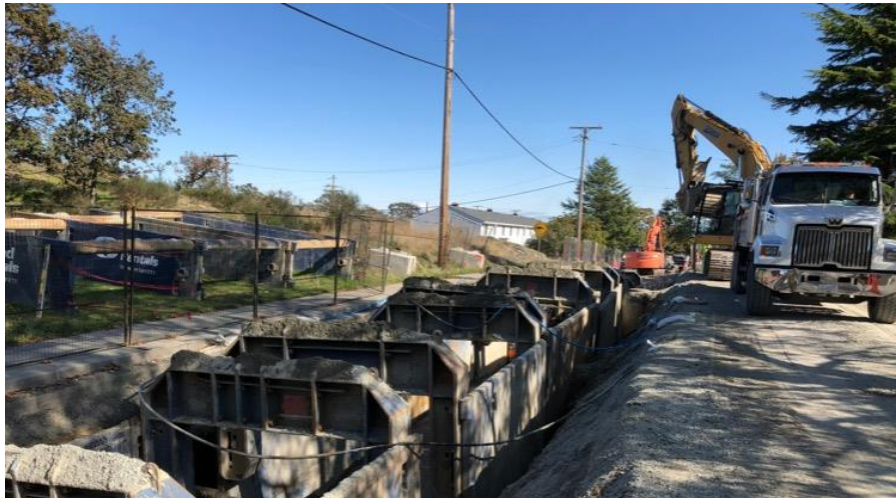
Figure 15-Macaulay Point Pump Station- Macaulay forcemain progressing east on Bewdley St to Peter St.
