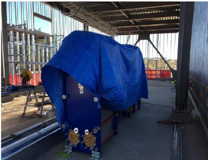
Figure 4- McLoughlin Point Wastewater Treatment Plant- Heat exchangers in Heat Recovery Room.
