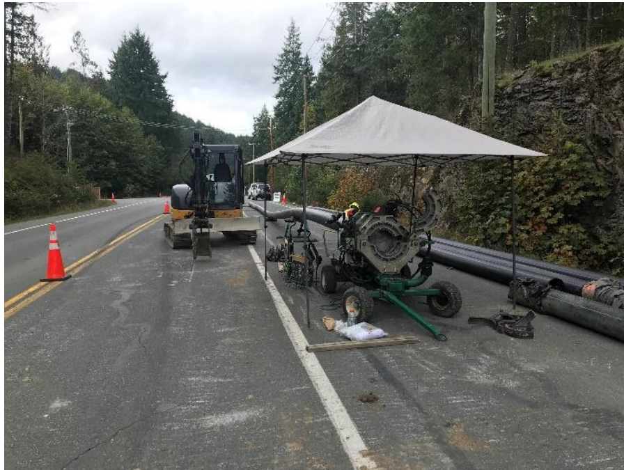
Figure 26 –Residual Solids Pump Stations and Bridge Crossings- Fusing of pipes on Willis Point Road.
