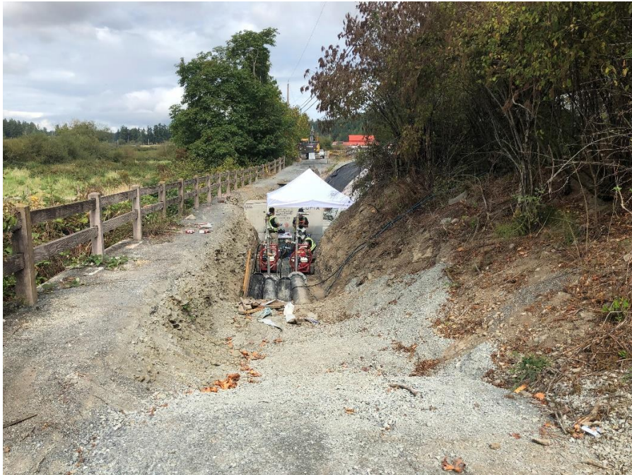
Figure 22–Residual Solids Conveyance Line- Pressure testing of pipe underway on Interurban Trail south of the Red Barn Market.
