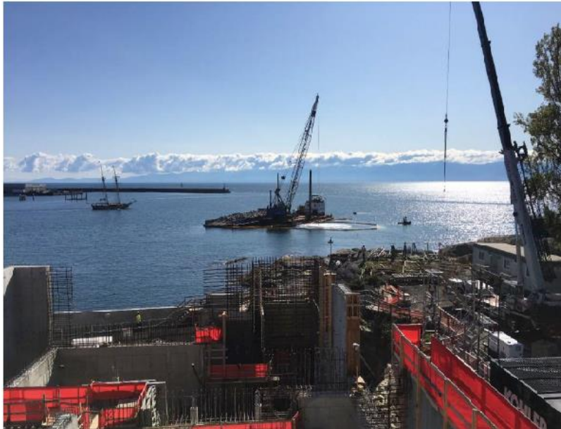
Figure 3- McLoughlin Point Wastewater Treatment Plant- Placement of Rip Rap on anchor protection zone.
