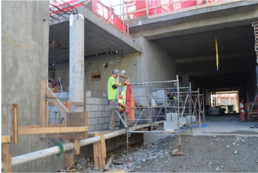
Figure 5– McLoughlin Point Wastewater Treatment Plant- Ongoing placement of concrete block at Operations and Maintenance building.
