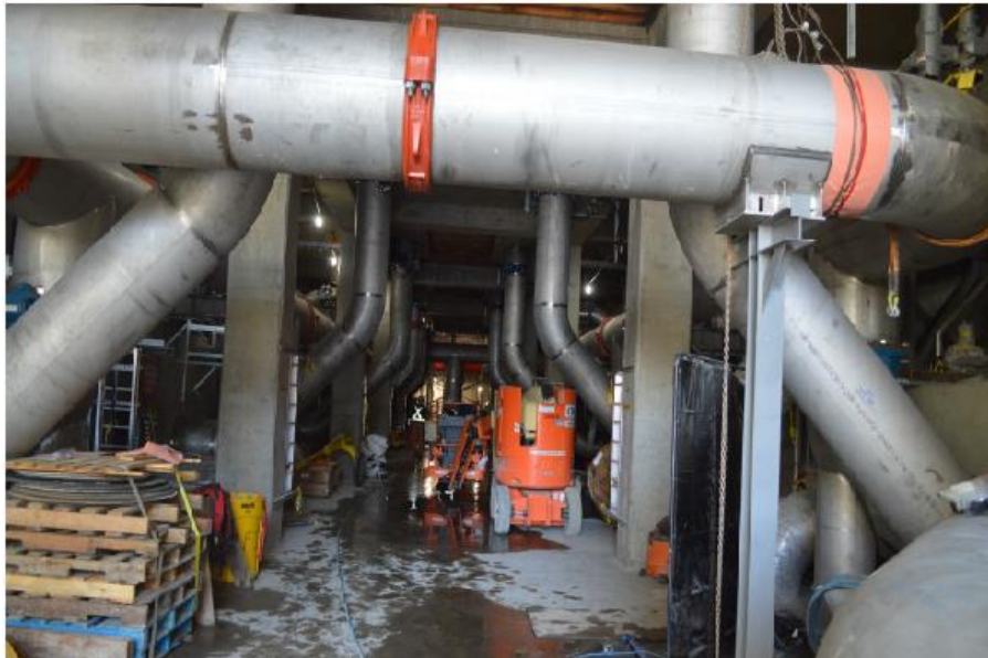
Figure 6– McLoughlin Point Wastewater Treatment Plant- Primary influent drop pipes from Biological Aerated Filter influent channel completed.
