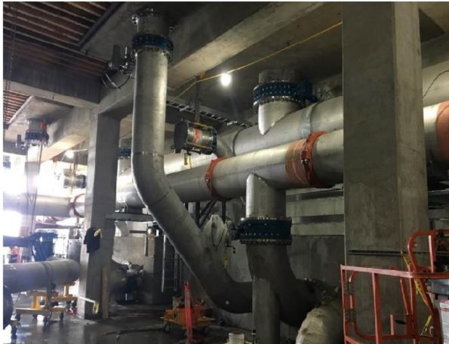
Figure 2– McLoughlin Point Wastewater Treatment Plant- Installing 24 inch Biological Aerated Filter influent piping.
