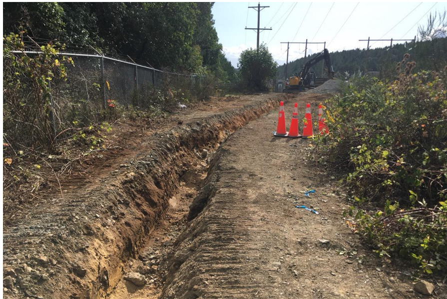
Figure 25–Residual Solids Pump Stations and Bridge Crossings – Excavation of trench to install Hartland water system improvements water main.
