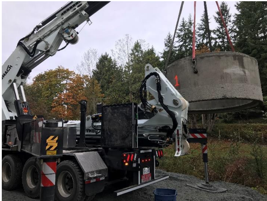
Figure 27–Residual Solids Pump Stations and Bridge Crossings – Crane truck offload 1500mm wet well barrel at pump station 3.
