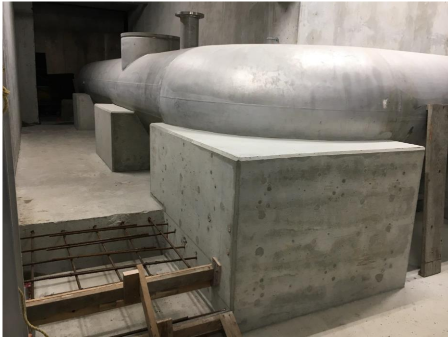
Figure 13–Clover Point Pump Station- Lower pump room concrete pipe supports.
