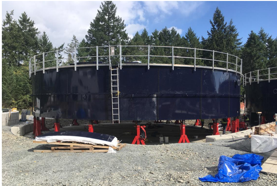
Figure 9– Residuals Treatment Facility- 3 rd row of bolted steel tank panels being installed on Residual Solids Tank 1.
