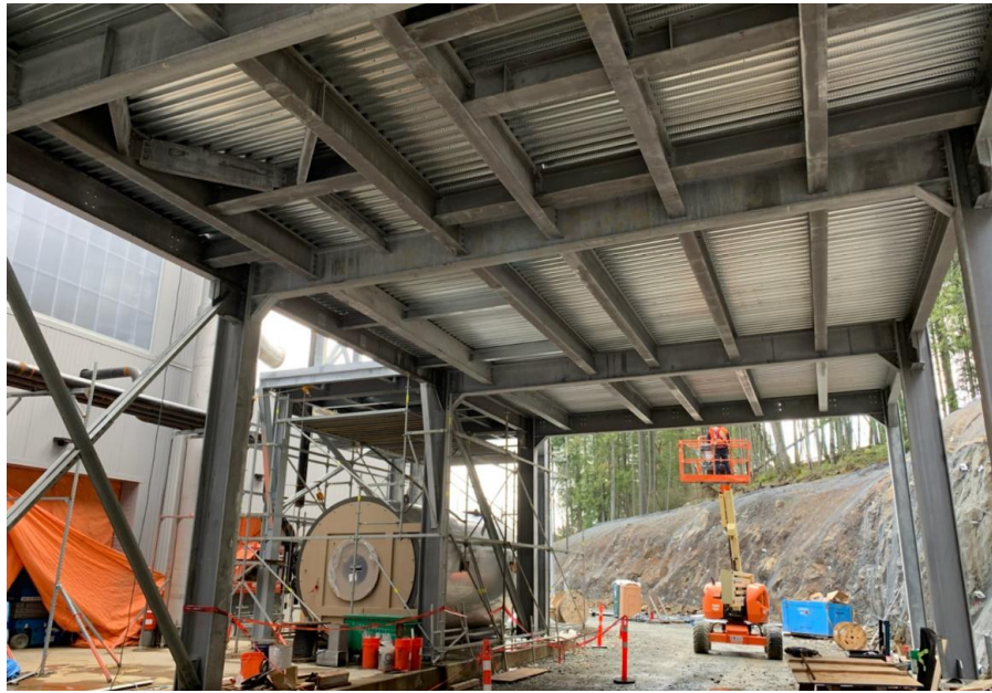
Figure 8– Residuals Treatment Facility- Installation of Q deck roofing system ongoing on product load out structure.
