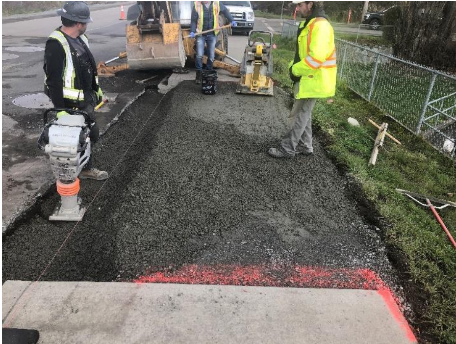
Figure 20– Residual Solids Pipes-Sidewalk, curb and gutter preparation on Interurban Road at Charlton Road
