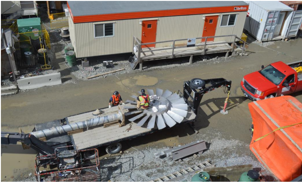
Figure 5– McLoughlin Point Wastewater Treatment Plant- delivery of turbine blade for Densadeg reactor.
