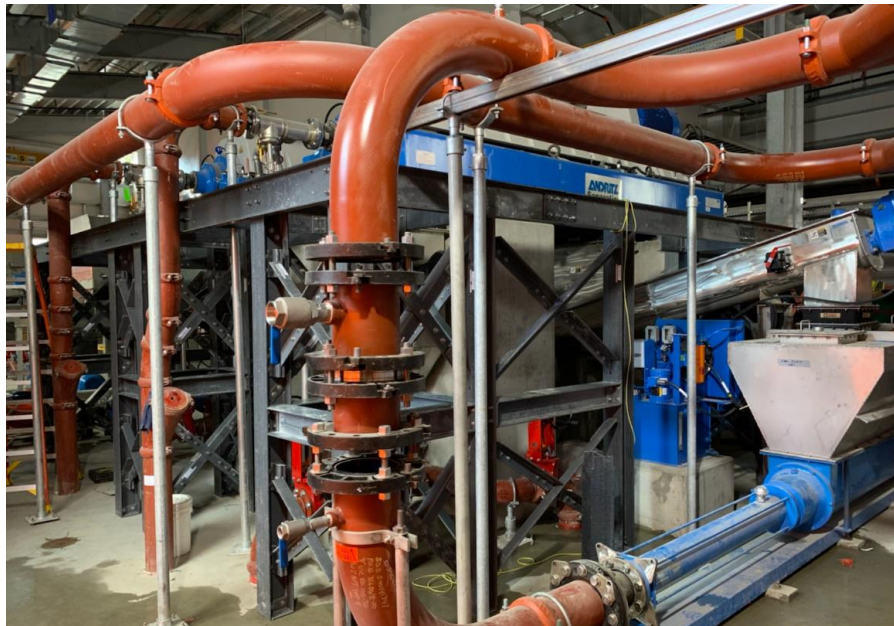
Figure 7– Residuals Treatment Facility- FRP supports being assembled for grating around centrifuges in Residuals Handling Building.
