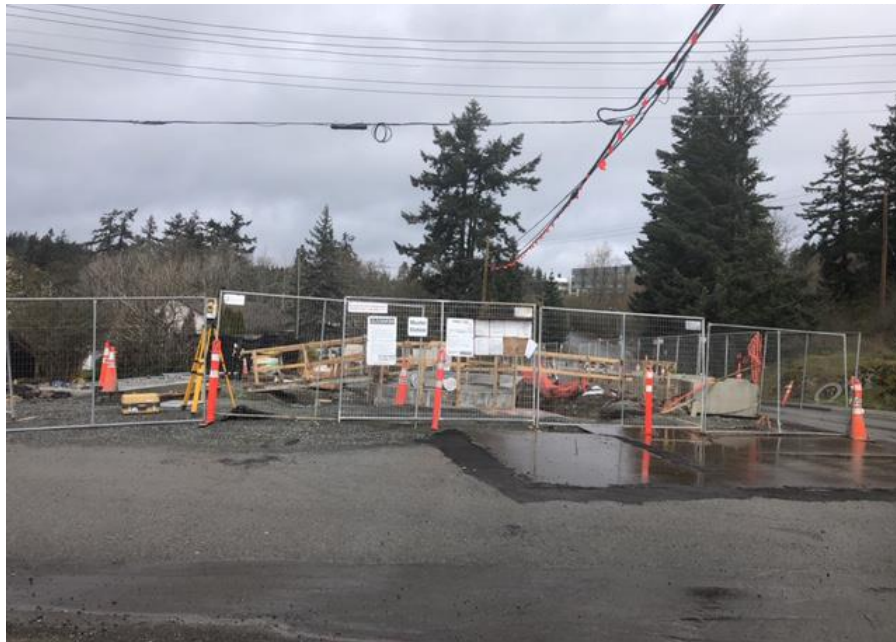
Figure 25 –Residual Solids Pump Stations – Pump Station1 Survey layout for generator and odour control unit pads.
