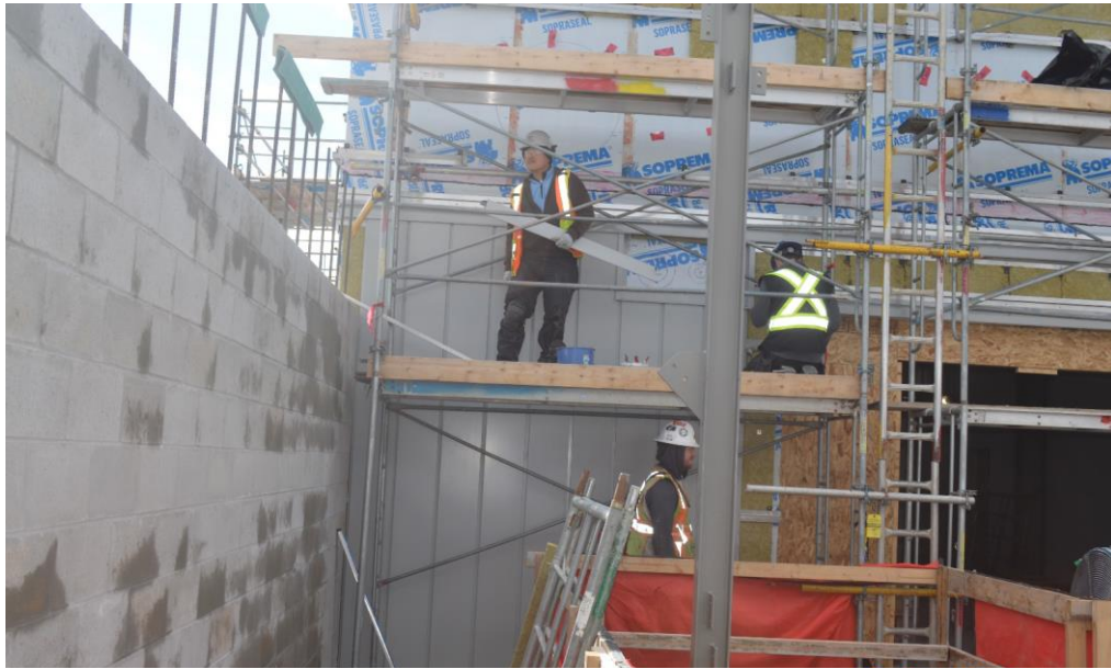
Figure 3- McLoughlin Point Wastewater Treatment Plant- Cladding installation on north end of heat recovery room.
