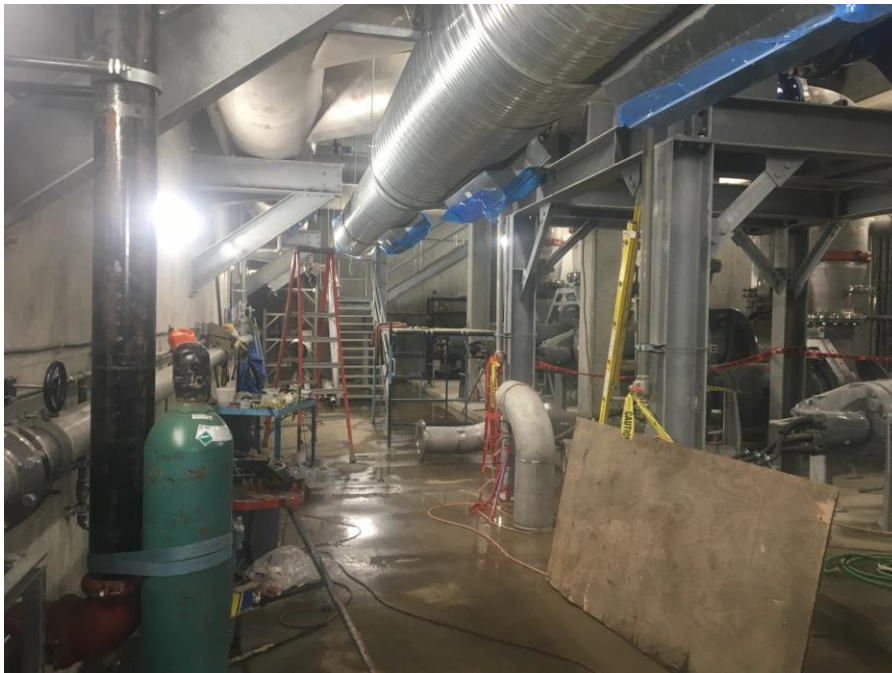
Figure 12–Clover Point Pump Station- Lower pump room
