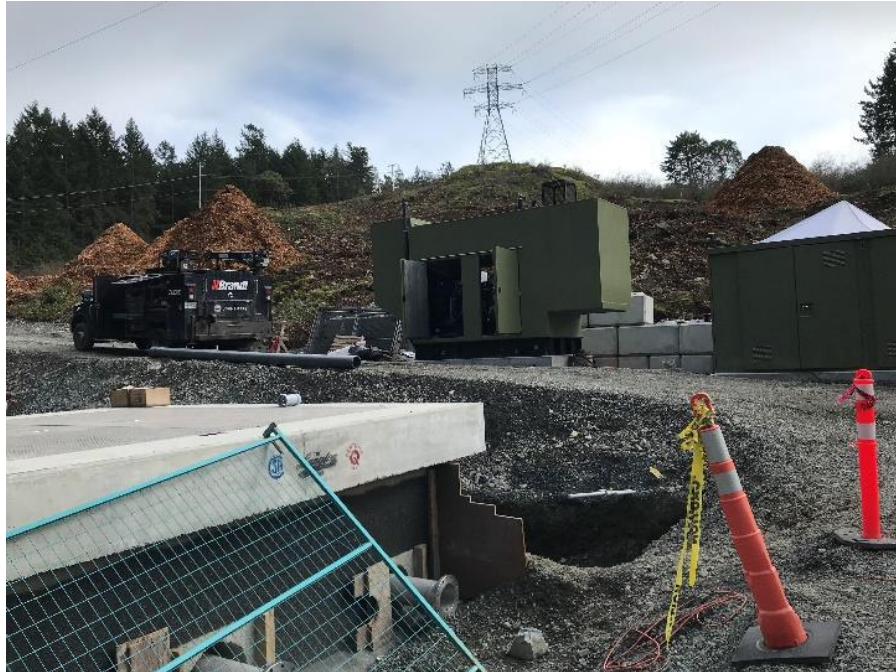
Figure 24–Residual Solids Pump Stations– Pump Station 3 – Emery Electric performing a 5– hour load test on the generator.
