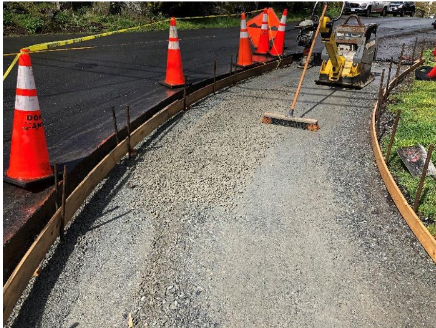
Figure 23–Residual Solids Pipes - Sidewalk, curb and gutter preparation on corner of Burnside Road and Grange Road.
