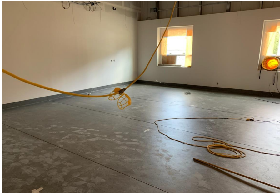
Figure 10– Residuals Treatment Facility – Interior painting and flooring installation ongoing in operations building
