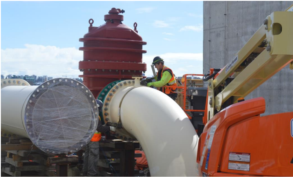
Figure 2– McLoughlin Point Wastewater Treatment Plant - Bolting up valve and fittings at pigging chamber preparing for pressure test.
