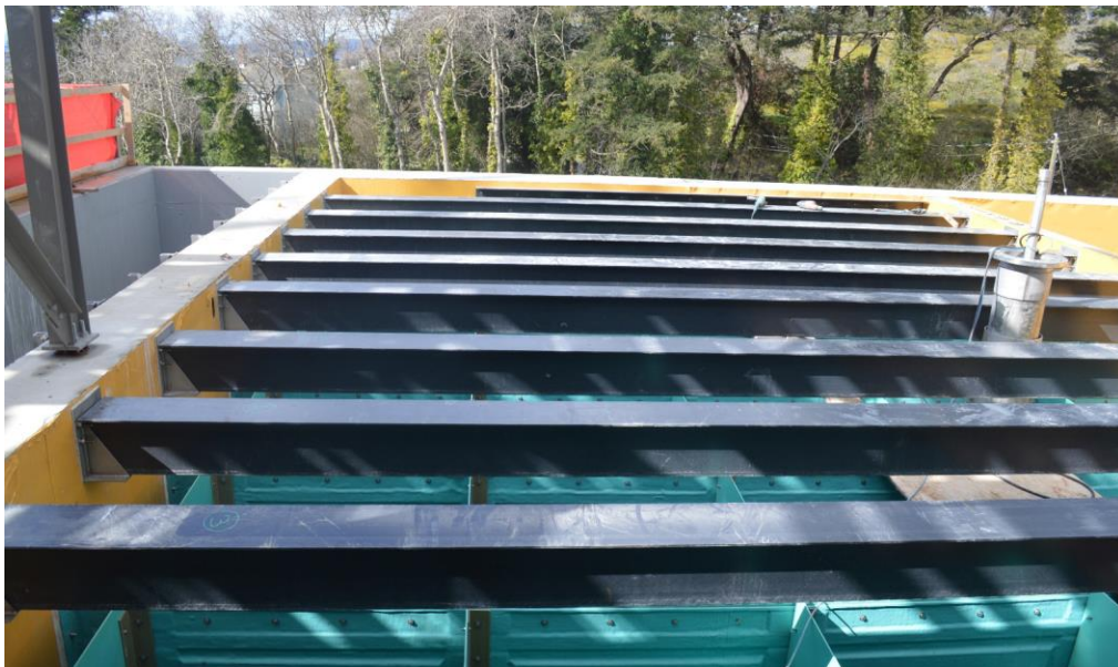
Figure 4- McLoughlin Point Wastewater Treatment Plant- Fibreglass reinforced plastic beams installed and ready for covers at DD3 final clarifier.
