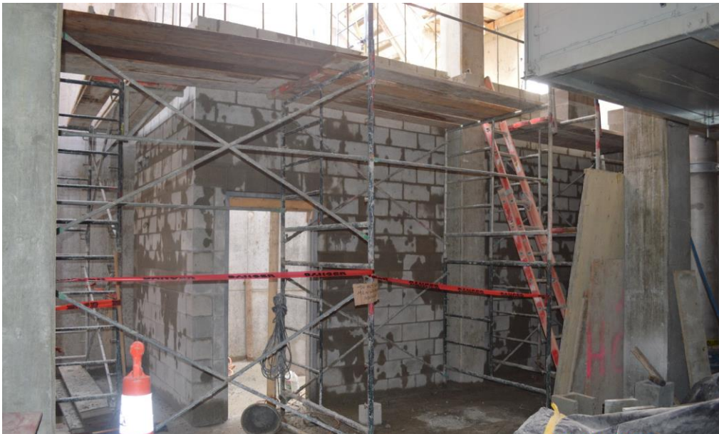
Figure 6– McLoughlin Point Wastewater Treatment Plant- Cinder block installation at northeast stairwell of tertiary treatment structure.
