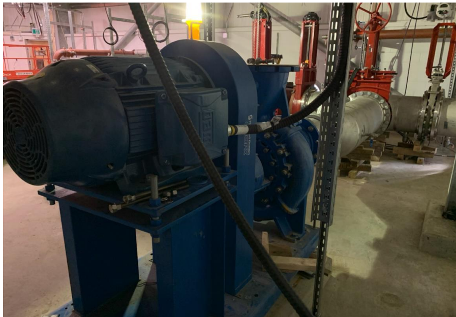
Figure 9– Residuals Treatment Facility- Chopper pumps wired in digester equipment building.
