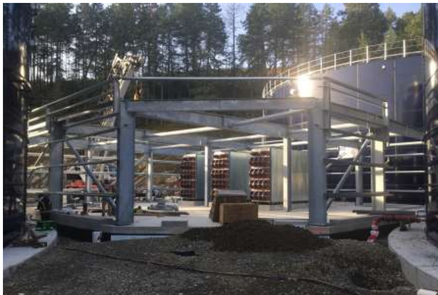
Figure 7– Residuals Treatment Facility- Installation of insulated metal cladding support members on Digester Equipment Building.
