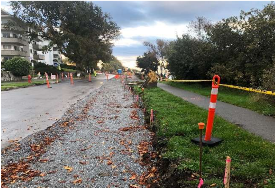
Figure 17–Clover Forcemain- Curb and gutter removals and base preparation along Dallas (South Side - Douglas to Government)
