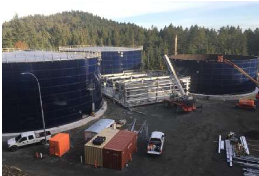
Figure 10– Residuals Treatment Facility- Digesters #1 and #2, Digested Solids Storage Tank and Digester Equipment Building.
