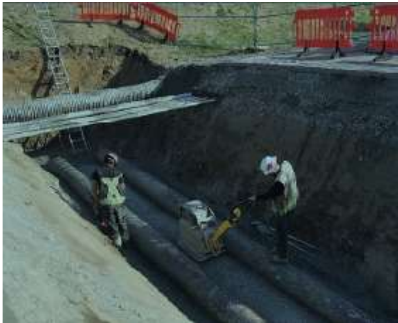
Figure 24–Residual Solids Conveyance Line- Backfill and compaction of highway crossing phase 3 pipe sleeves.
