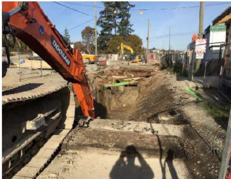
Figure 3– McLoughlin Point Wastewater Treatment Plant- Excavation of Macaulay forcemain pipe trench on Victoria View Road
