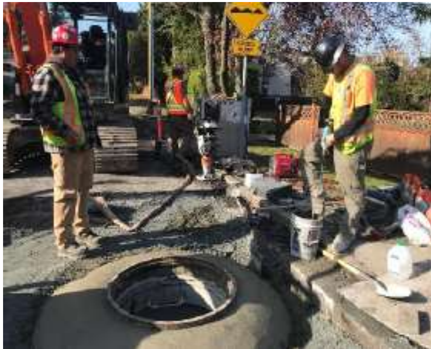
Figure 23-Residual Solids Conveyance Line- Placing concrete around manhole grade rings and frame on Selkirk Ave
