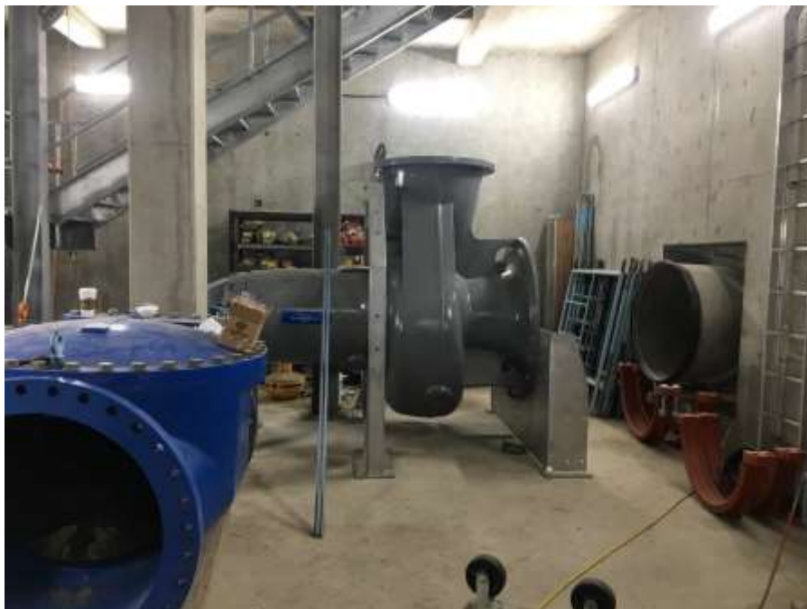
Figure 11–Clover Point Pump Station- Storm pump.
