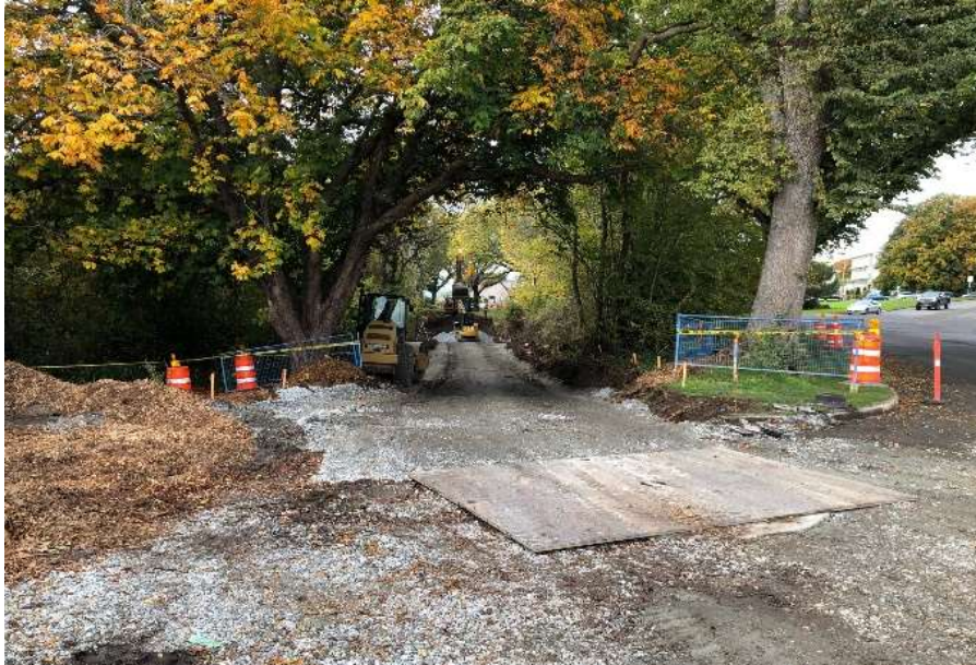
Figure 18–Clover Forcemain- Cycle track sub-grade excavation and sub-base & base grade development along corridor at the foot of Douglas.
