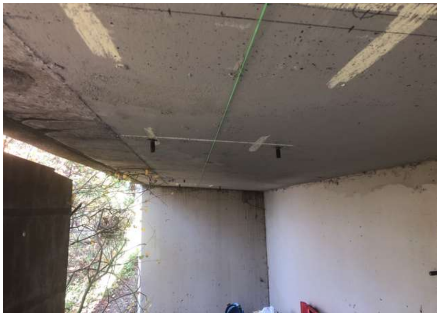
Figure 27–Residual Solids Pump Stations and Bridge Crossings – Commence pipe hanger installation at Tillicum Bridge.
