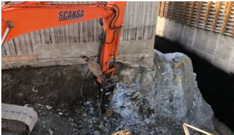
Figure 15–Macaulay Point Pump Station- Rock removal between diversion chamber and existing pump station.
