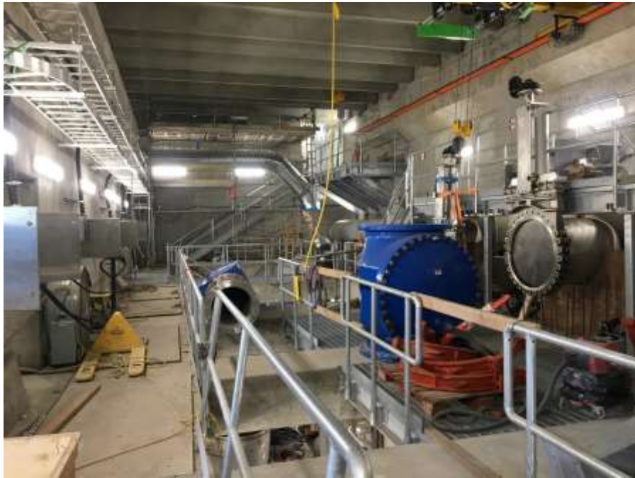
Figure 12–Clover Point Pump Station- upper pump room.
