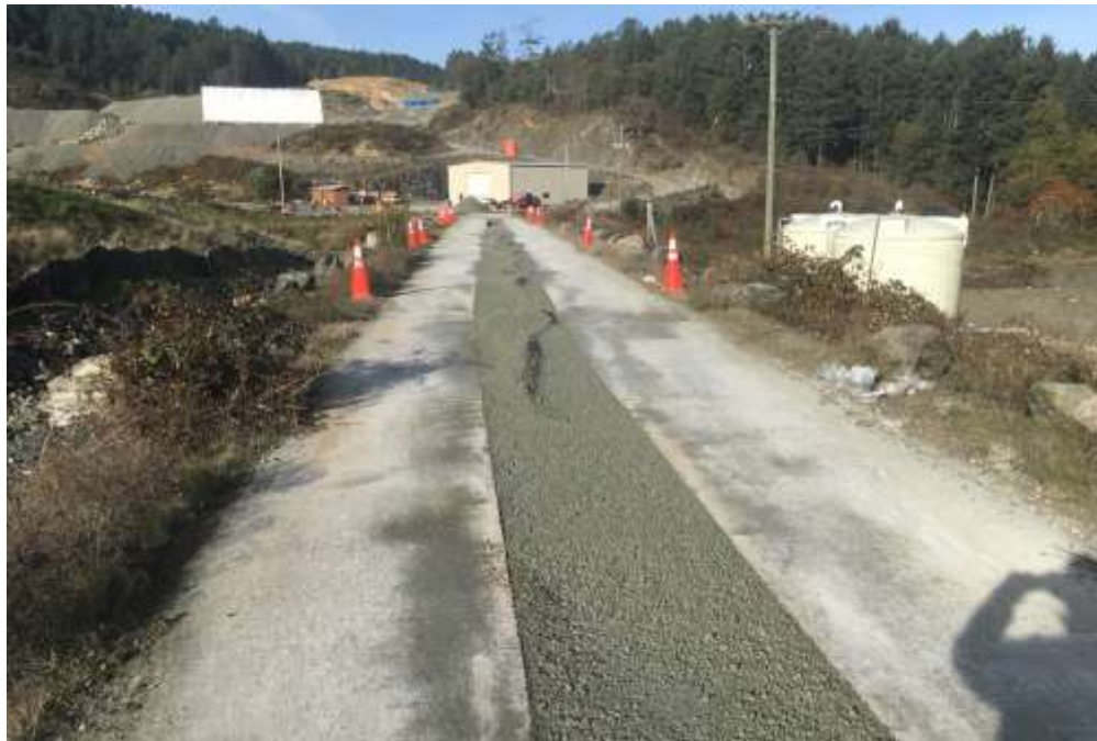
Figure 25–Residual Solids Pump Stations and Bridge Crossings – Watermain trench backfilled west of gas plant.
