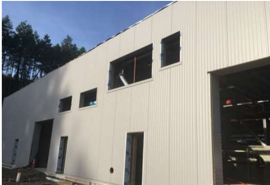
Figure 8- Residuals Treatment Facility- Installation of flashing around wall penetrations on east side of Residuals Handling Building
