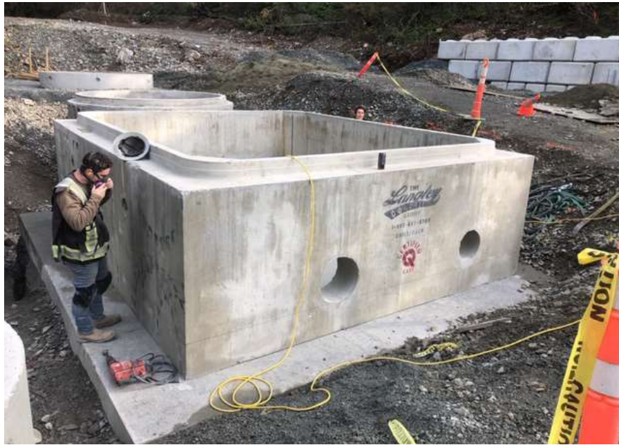
Figure 26 –Residual Solids Pump Stations and Bridge Crossings- Installed pre-cast valve chamber at Pump Station 3
