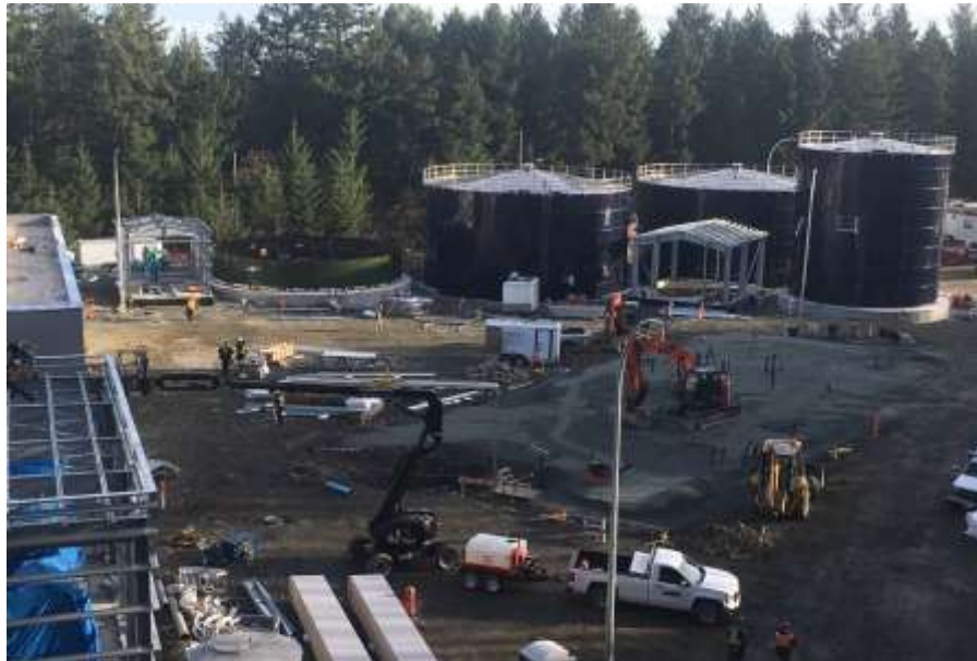
Figure 9- Residuals Treatment Facility- Site overview showing Residuals Solids Tanks, Effluent Tank, Water Storage Tank, Equalization Building and Water Pump House.
