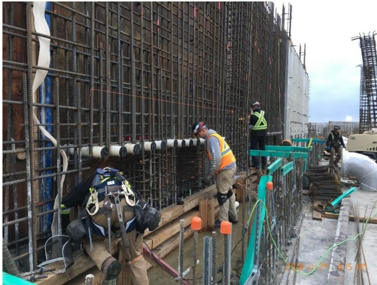
Figure 2 – McLoughlin Point Wastewater Treatment Plant: installing rebar couplers in biological aerated filter (BAF) wall 19.
