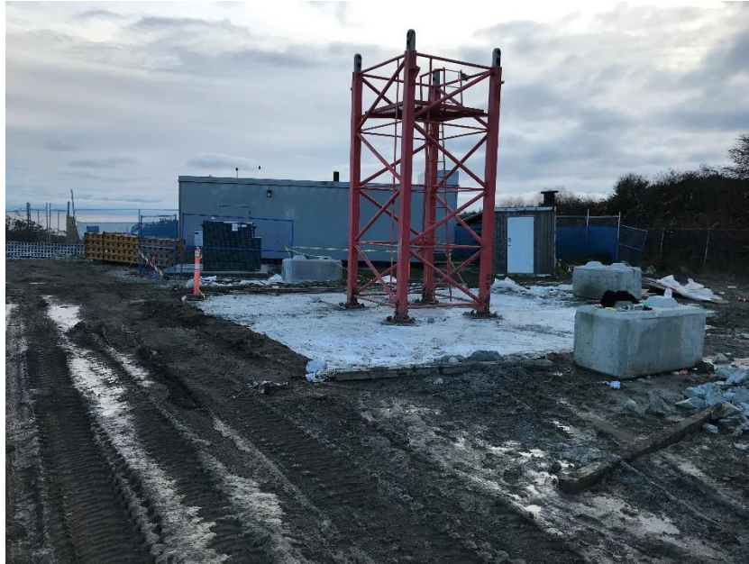
Figure 19 – Macaulay Point Pump Station: tower crane base poured and crane erection commenced.
