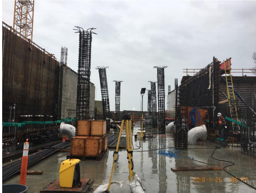
Figure 5 – McLoughlin Point Wastewater Treatment Plant: standing column steel in biological aerated filter (BAF) gallery.
