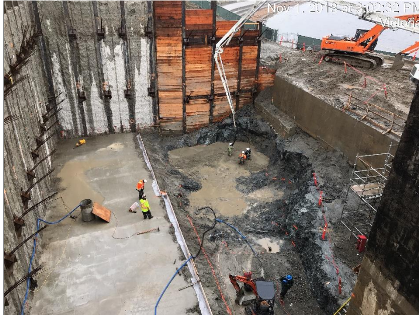
Figure 16 – Clover Point Pump Station: placing mud slab in the storm wet well area.
