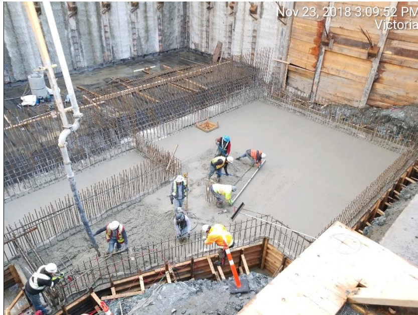
Figure 14 – Clover Point Pump Station: placing and finishing concrete at sanitary and storm wet well slabs.
