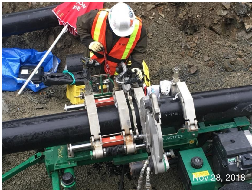
Figure 9 – Residuals Treatment Facility: fusion bonding of the Residual Solids Conveyance Line in progress.
