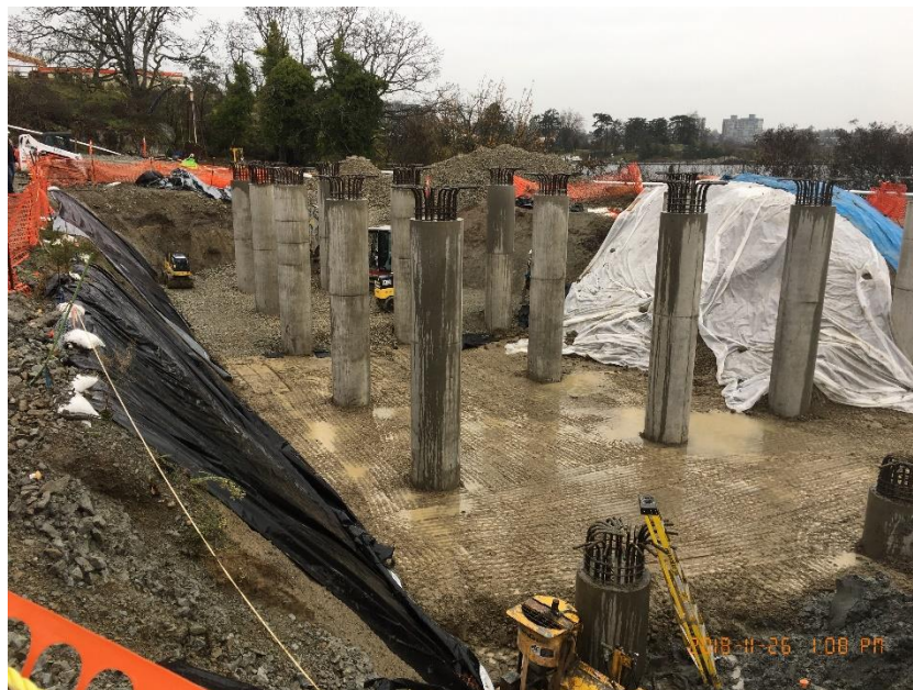
Figure 6 – McLoughlin Point Wastewater Treatment Plant: backfilling and compacting in the Odour Control excavation.
