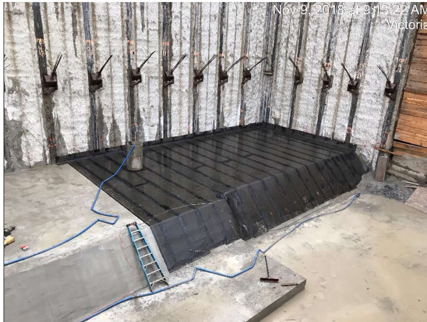
Figure 17 – Clover Point Pump Station: installation of waterproofing membrane on pump room mud slab.
