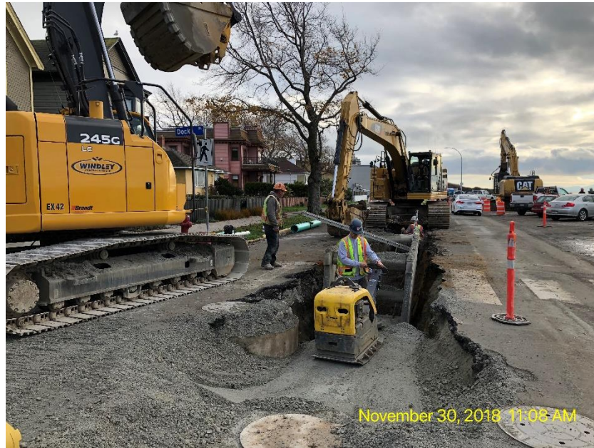
Figure 22 – Clover Forcemain: Dallas Road at Dock Street, trench backfill and compaction east of installed sanitary manhole B.
