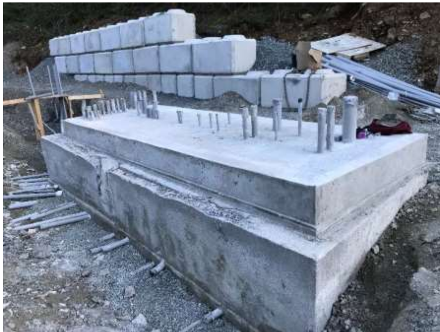
Figure 25–Residual Solids Pump Stations and Bridge Crossings – Pump Station 4 – grinding kiosk slab to level.
