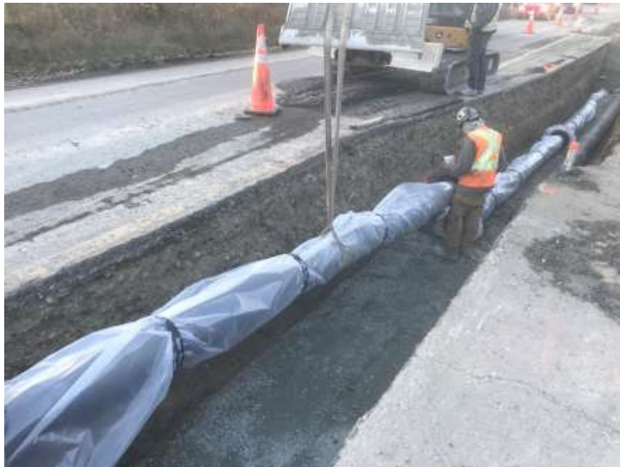
Figure 23–Residual Solids Conveyance Line- Ductile iron pipe installation on Interurban Rd near North Road.
