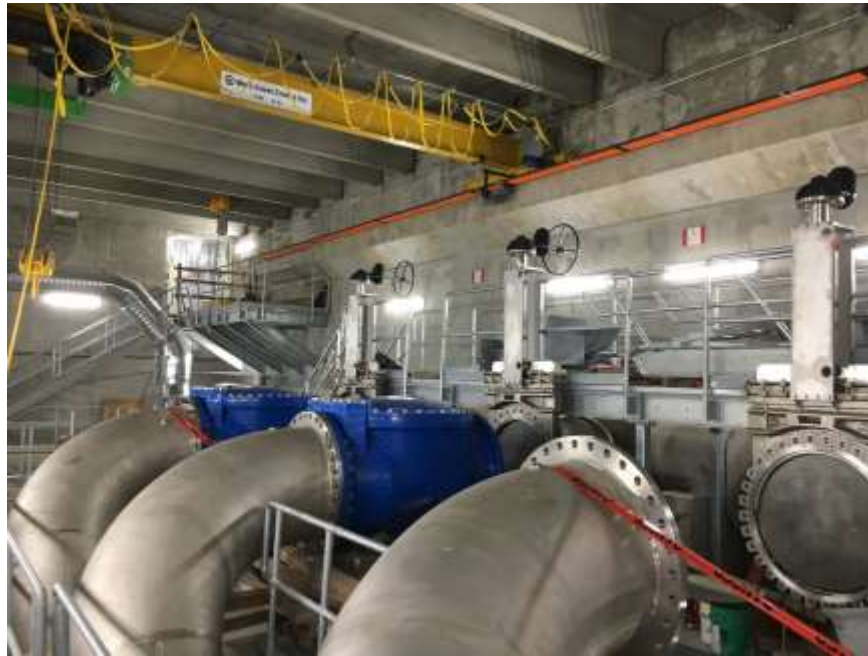
Figure 12–Clover Point Pump Station- Upper pump room.
