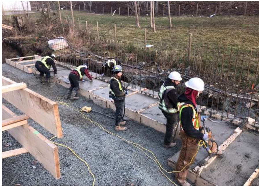
Figure 26 –Residual Solids Pump Stations and Bridge Crossings- Placing concrete in Pump Station 3 South East retaining wall footing.
