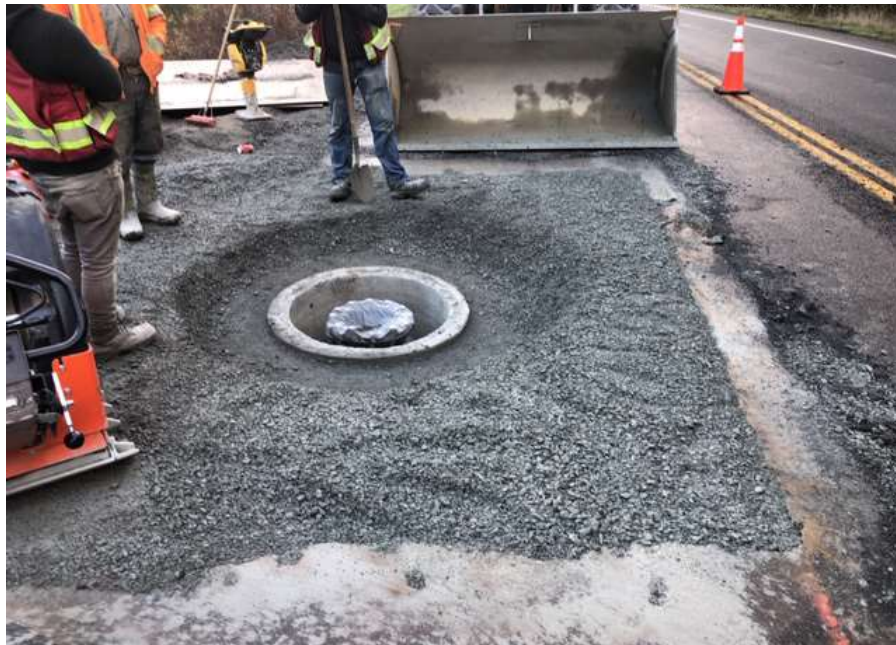
Figure 27–Residual Solids Pump Stations and Bridge Crossings – Backfilled cleanout on Willis Point Road.
