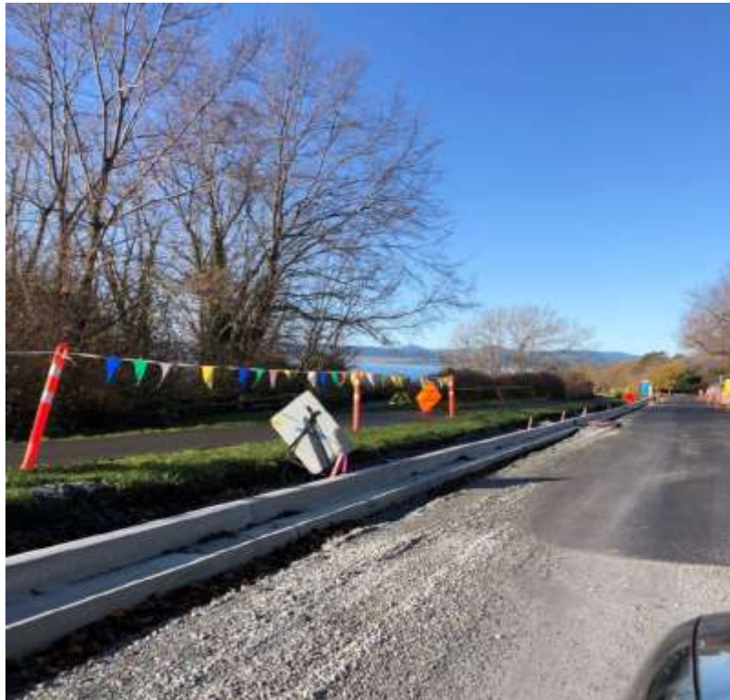
Figure 19–Clover Forcemain– Cycle track and road restoration between Douglas Street and Government Street.
