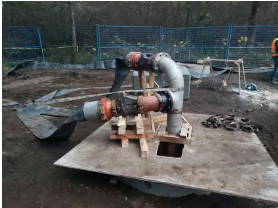
Figure 29– Arbutus Attenuation Tank –Bypass pumping delivery header.
