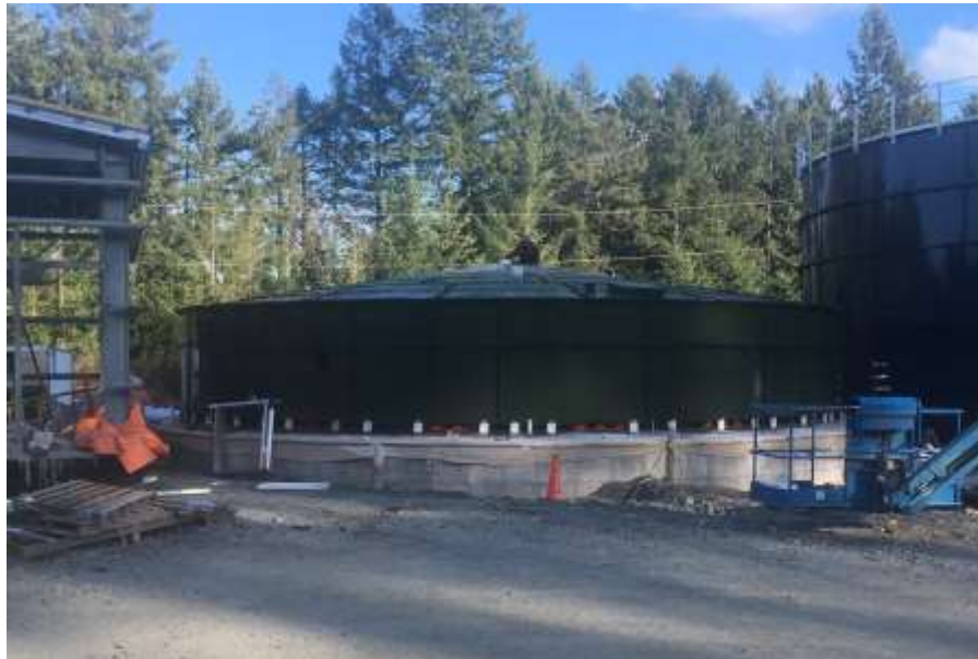
Figure 7- Residuals Treatment Facility- Installation of bolted steel roof panels on water storage tank.
