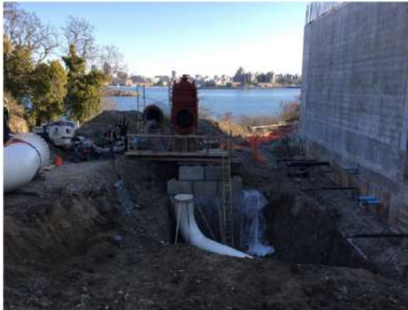
Figure 2– McLoughlin Point Wastewater Treatment Plant- Installation of pig receiver station, piping and valves.
