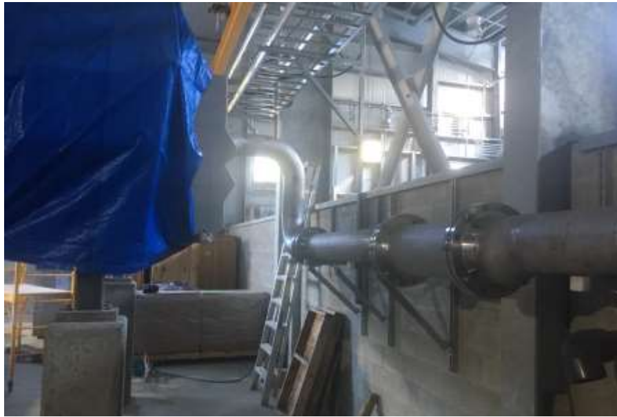
Figure 9– Residuals Treatment Facility- Installation of stainless steel process piping ongoing in Residuals Handling Building.
