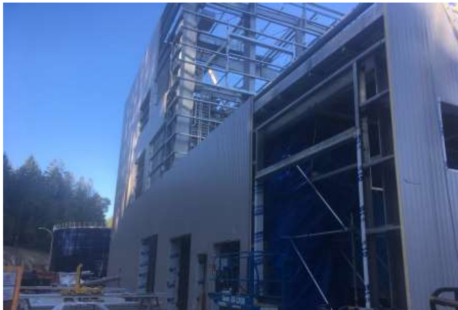
Figure 10– Residuals Treatment Facility- Installation of insulated metal cladding panels on south side of Dryer Building.
