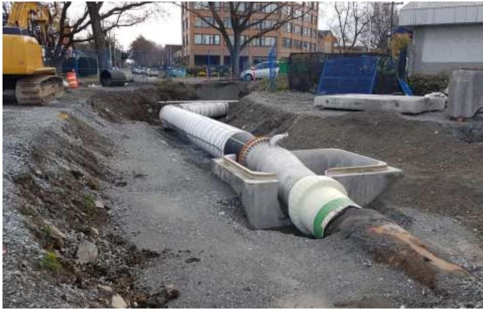
Figure 17–Clover Forcemain- Final tie-in to the Harbour Crossing pipe in the transition chamber.
