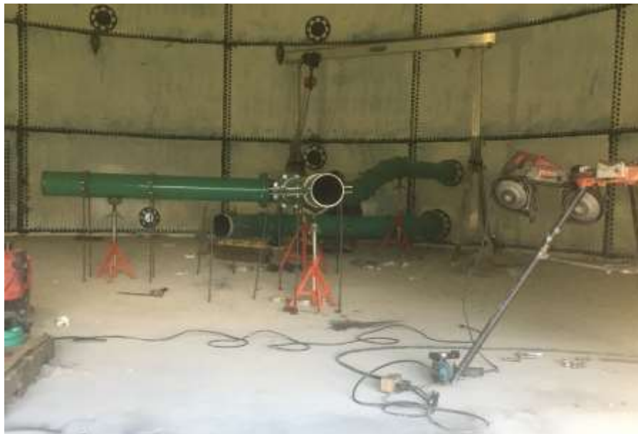
Figure 8- Residuals Treatment Facility- Glass lined and coated ductile iron process piping being installed in effluent tank.
