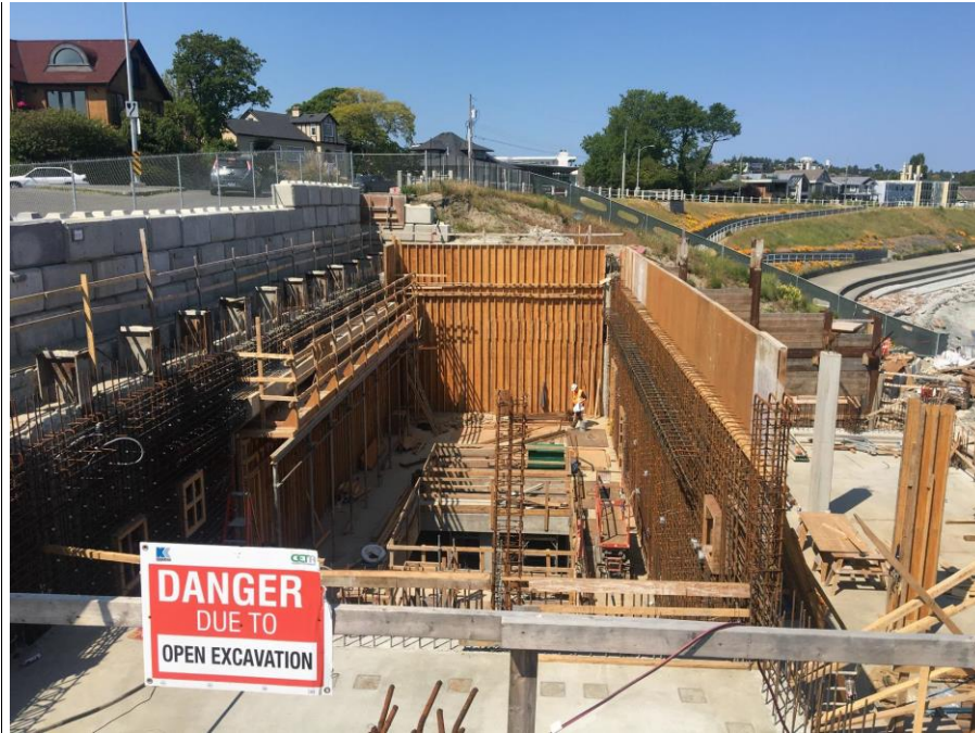
Figure 14 –Clover Point Pump Station – site overview looking north.
