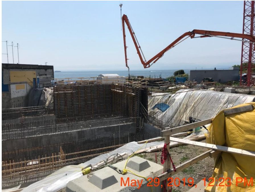
Figure 19 – Macaulay pump station & forcemain – pouring the second lift of the exterior wall SW corner.
