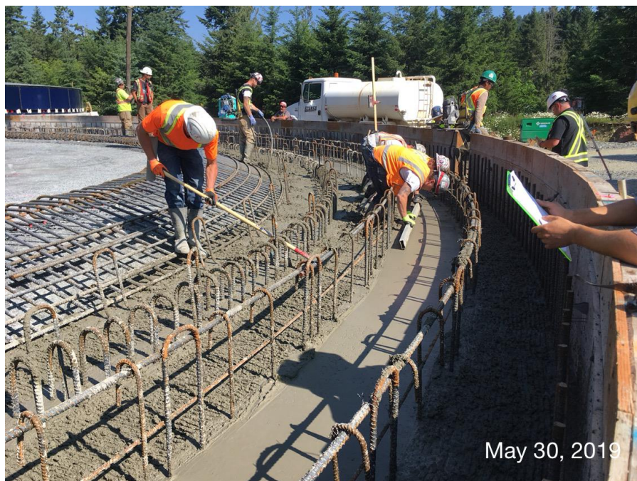
Figure 10 - Residuals Treatment Facility – Concrete placement and finishing for digested sludge storage tank slab first pour.
