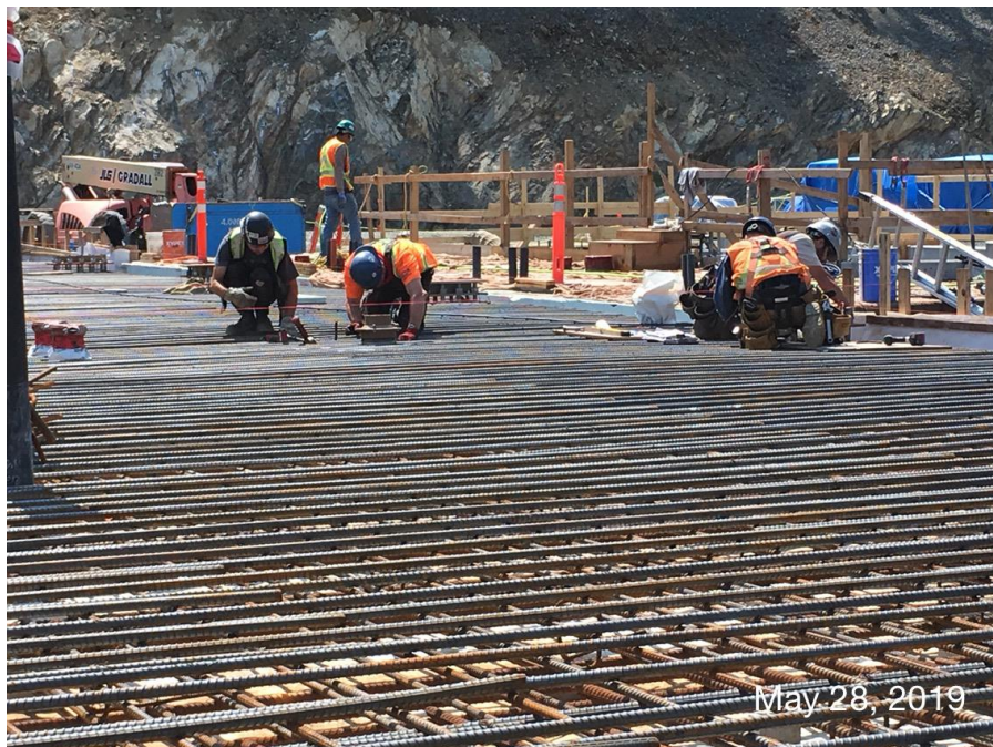
Figure 12 –Residuals Treatment Facility – Crew installing floor drains for residuals handling building prior to concrete floor slab pour.
