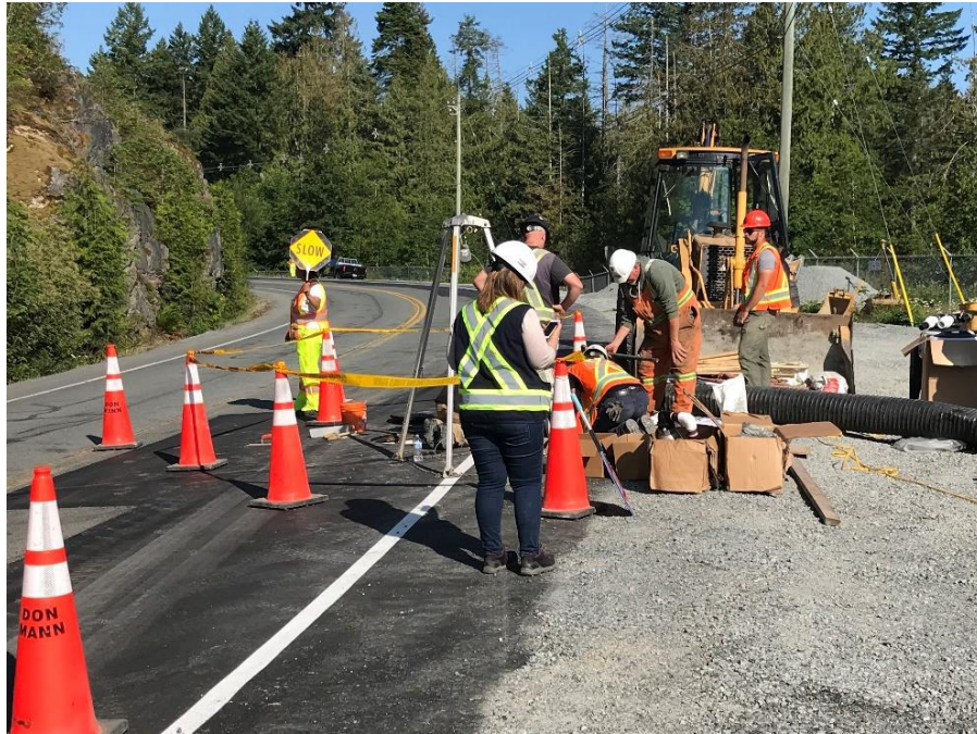
Figure 24 – RSCL 100: – Installing equipment inside the Air Valve Chamber on Willis Point Road.
