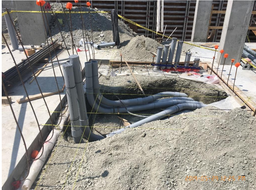
Figure 7 – Mcloughlin Point Wastewater Treatment Plant – installing conduit for Operations & Maintenance building electrical room.
