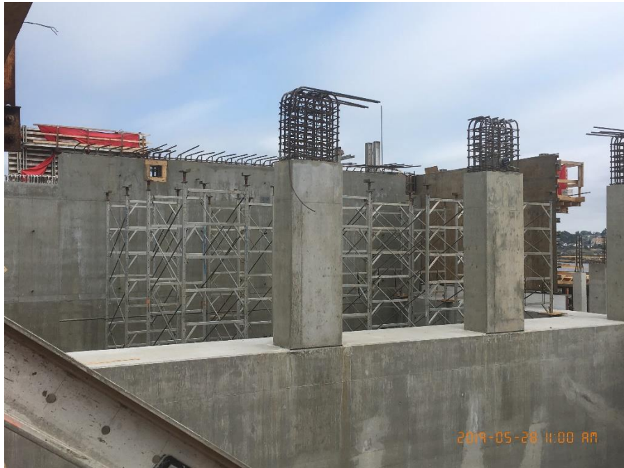
Figure 8 – Mcloughlin Point Wastewater Treatment Plant – Installing scaffolding for heat recovery room suspended slab.
