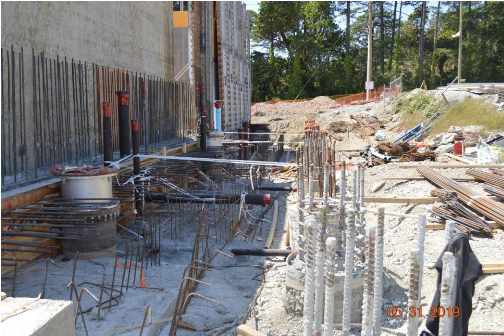
Figure 2 – Mcloughlin Point Wastewater Treatment Plant – Phase 3 piling completed at pump room at north end of Lamella plate settlers.
