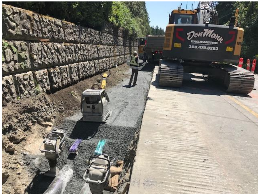
Figure 25 – RSCL100: - Minimum 150mm of pipe bedding placed in rock removal area on Interurban Road.
