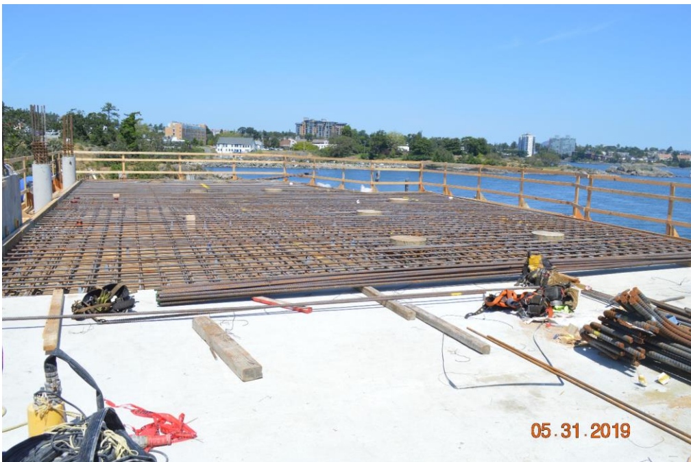
Figure 3 - Mcloughlin Point Wastewater Treatment Plant – Rebar completed for Operations & Maintenance building level 2 suspended slab pour
