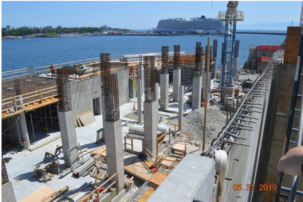
Figure 5 – Mcloughlin Point Wastewater Treatment Plant – Operations & Maintenance building looking SE from top of Densadeg No. 1.
