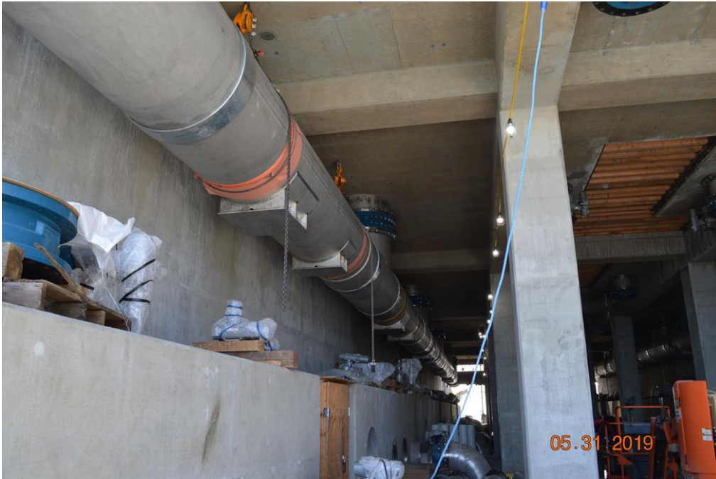
Figure 4 – Mcloughlin Point Wastewater Treatment Plant – 42" BWW header
