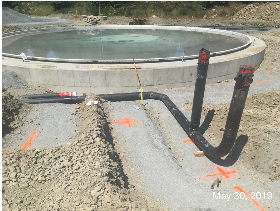
Figure 11– Residuals Treatment Facility – high density polyethylene process piping assembly installed at south side of residual solids.
