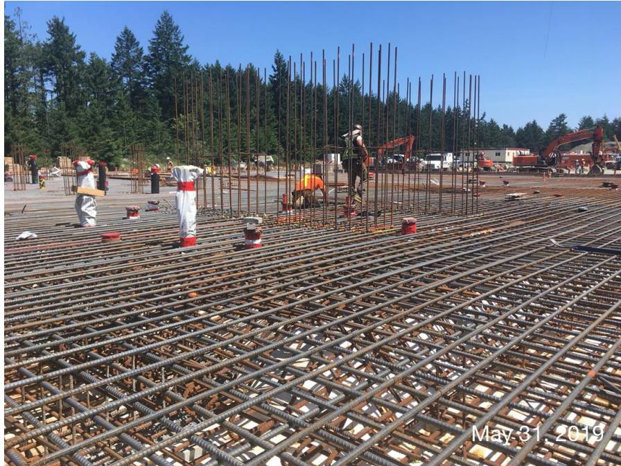
Figure 9– Residuals Treatment Facility – installation of reinforcing steel for Residuals Handling Building slab..
