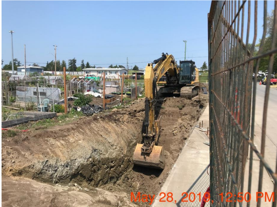
Figure 20 – Macaulay pump station & forcemain – trench excavation for Macaulay forcemain on Anson Street.
