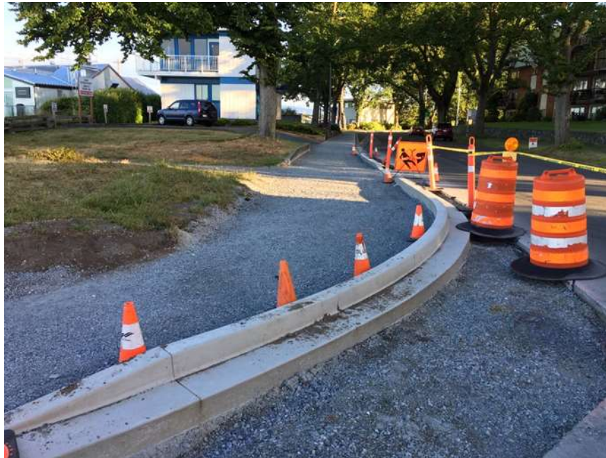
Figure 14–Clover Forcemain- Curb and gutter and sidewalk prep at Dock Street and Dallas road looking west.
