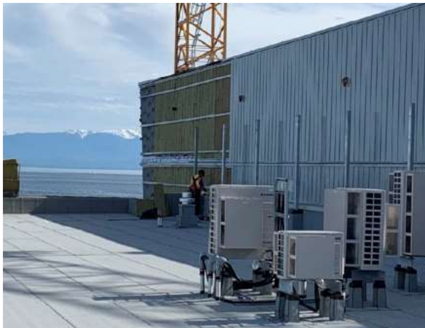
Figure 5- McLoughlin Point Wastewater Treatment Plant- Installing insulation and cladding on east face of Blower Building.
