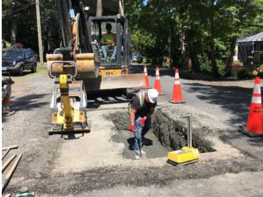
Figure 17-Residual Solids Pipes- Back fill and compaction on Grange Road after coupler repair.
