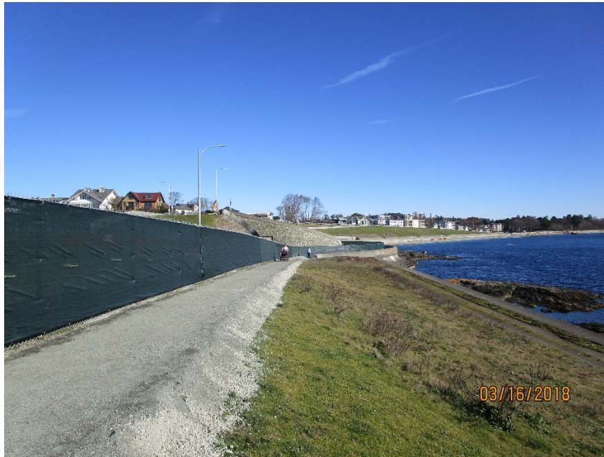
Figure 11 – View of pedestrian walkway – is the temporary walkway built for the public to walk beside the construction site.
