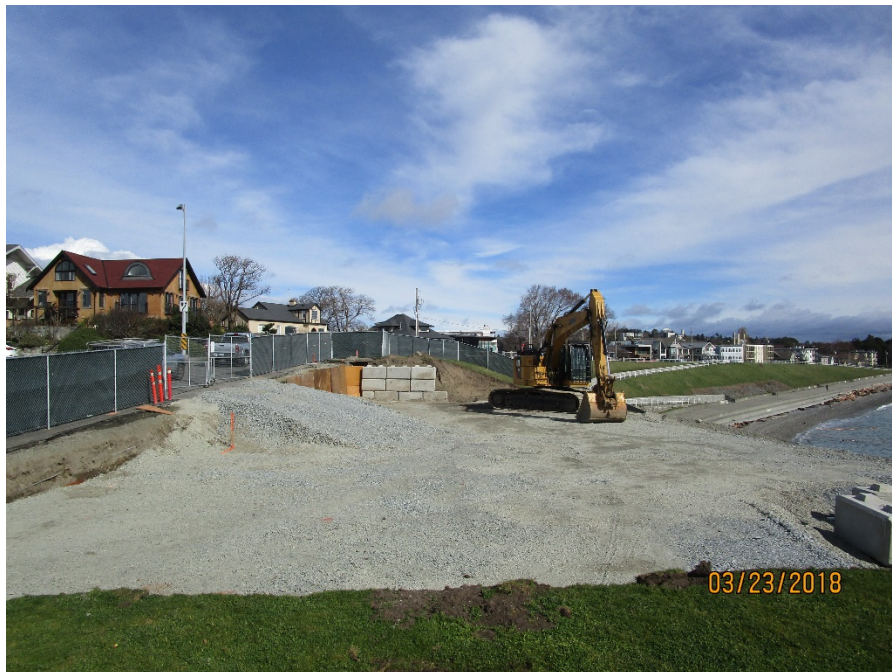
Figure 9 – General view looking north is the work area for the secant pile contractor.
