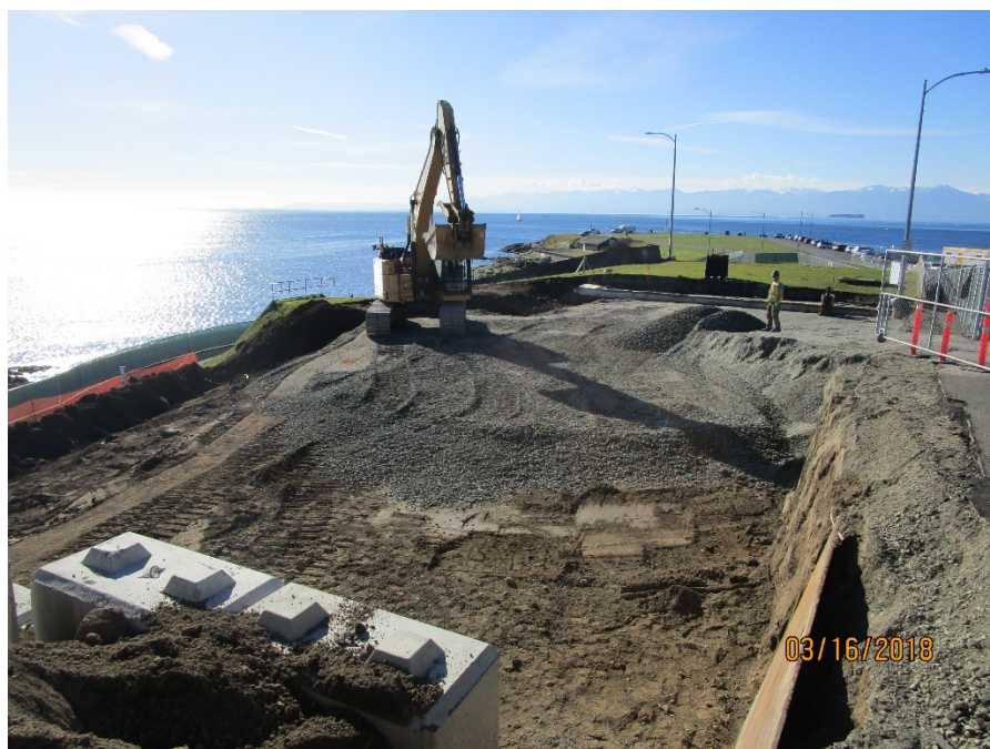
Figure 10 – Scansa progressing at future caisson mat – is the construction of the secant pile contractor work area.
