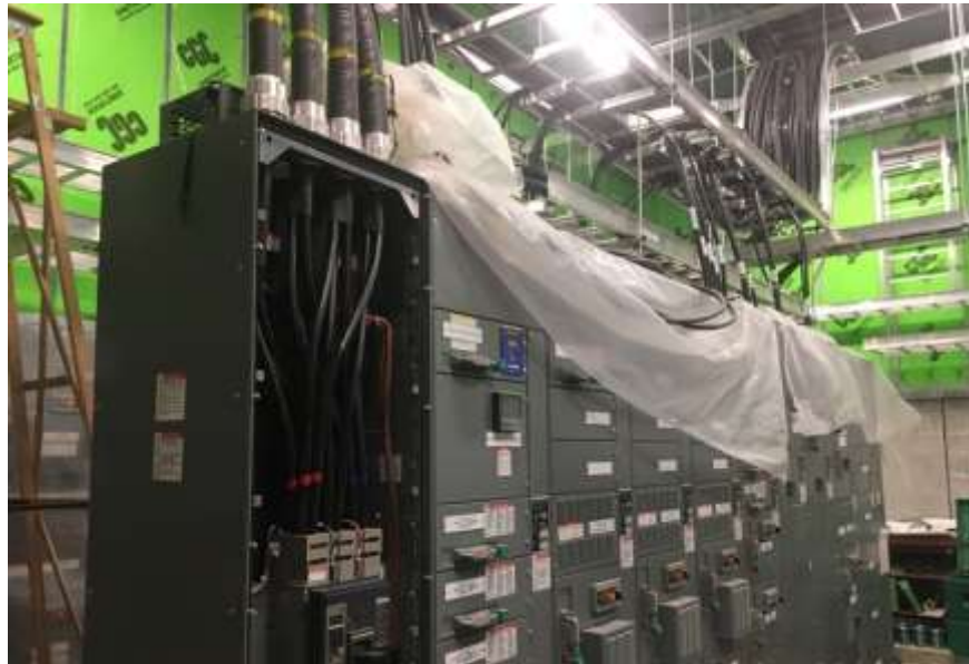
Figure 7– Residuals Treatment Facility- Residuals Handling building electrical room motor control centres.
