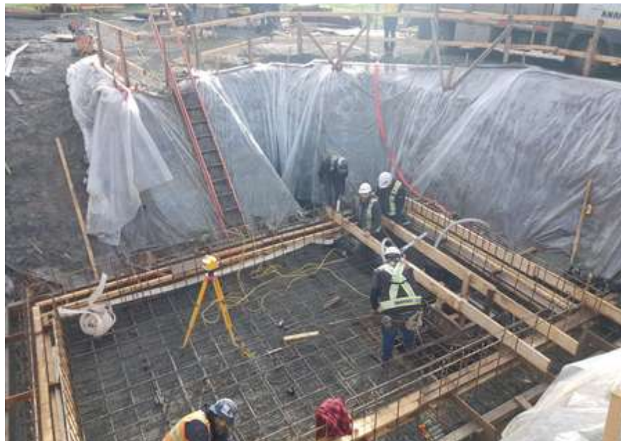
Figure 27–Residual Solids Pump Stations – Installing formwork and reinforcing steel for Marigold pump station valve chamber.
