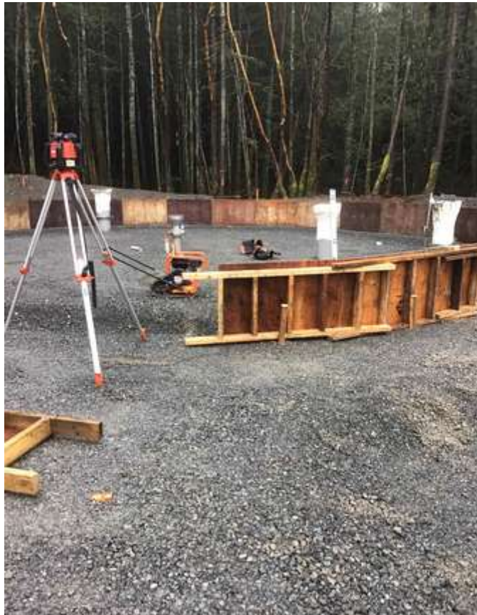
Figure 25–Residual Solids Pump Stations– Hartland Water System Improvements – Installation of formwork for the reservoir slab.
