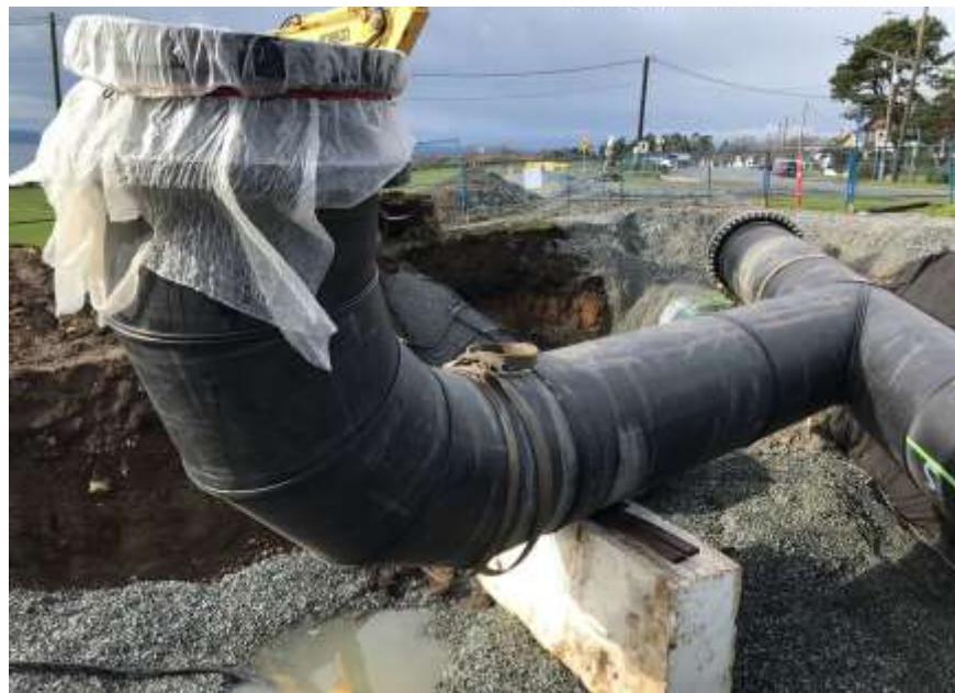
Figure 13–Clover Point Pump Station- Forcemain blind flange is installed and pigging station pipe bedding is being placed.
