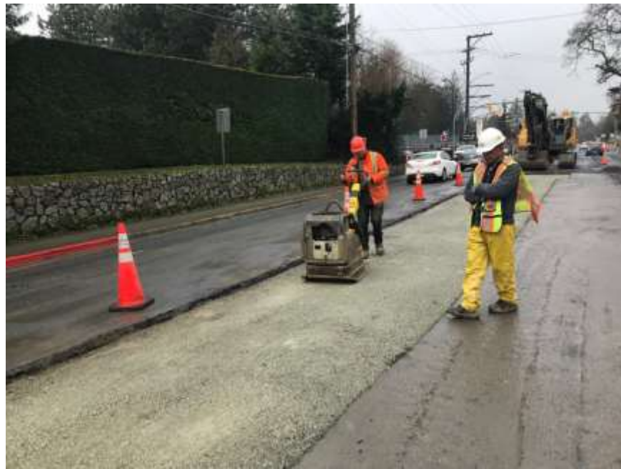
Figure 24–Residual Solids Pipes - Compaction being completed on prep work for temporary paving on Interurban Road.
