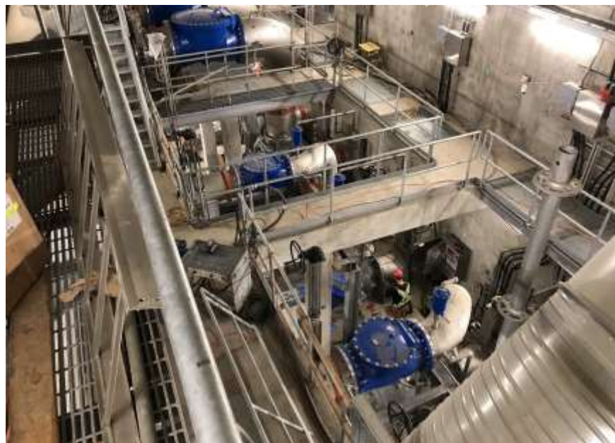
Figure 11–Clover Point Pump Station- Over the upper and lower pump rooms.
