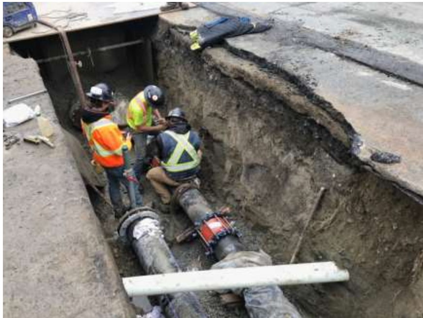
Figure 23–Residual Solids Pipes – Pipe Tie in at Interurban Road just south of Wilkinson Road.
