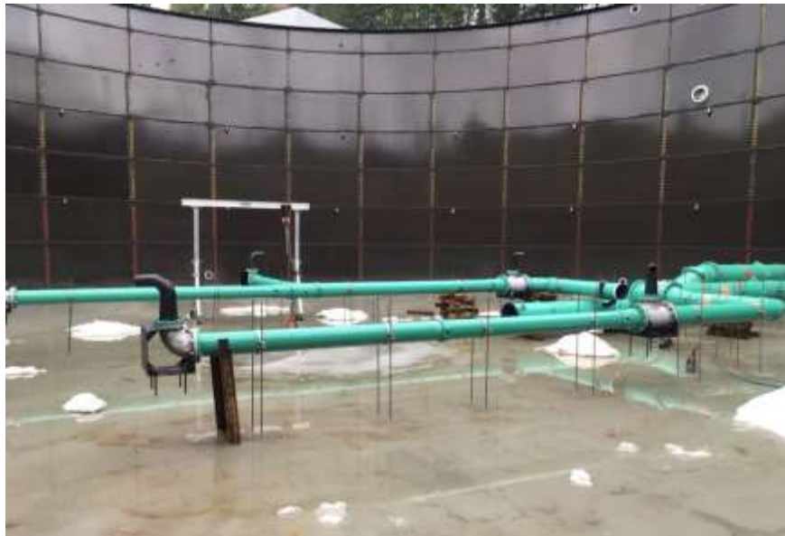
Figure 9– Residuals Treatment Facility- Digested Sludge Storage Tank process pipe and mix nozzles.
