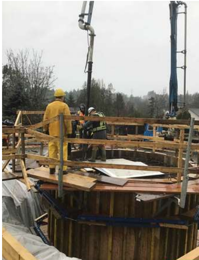
Figure 26 –Residual Solids Pump Stations - Pump Station 1- Wet well concrete pour in progress.
