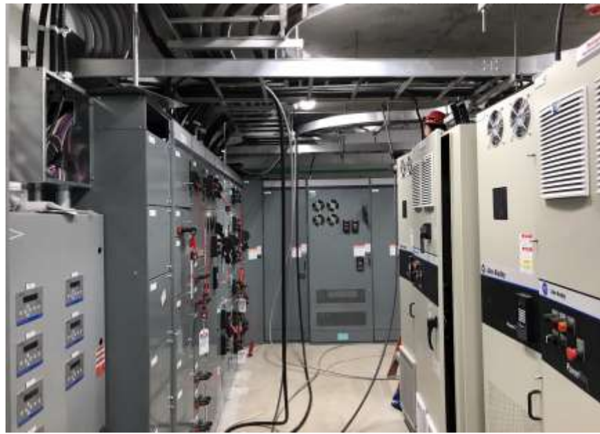
Figure 12–Clover Point Pump Station- Inside the electrical room.
