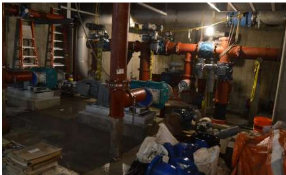
Figure 4- McLoughlin Point Wastewater Treatment Plant- Pumps and piping in the pump room.
