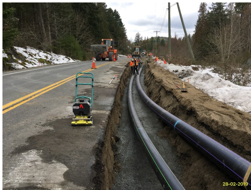
Figure 24 – RSCL: Segment 4 - installation of residual solids forcemain and centrate return line at Willis Point Road.
