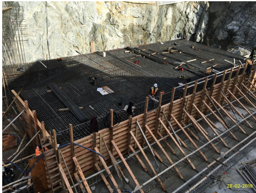
Figure 19 – Macaulay Point Pump Station: formwork and rebar for last base slab pour.
