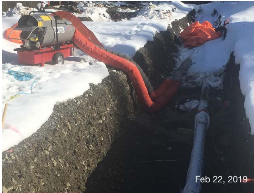
Figure 12 – Residuals Treatment Facility: heaters and tarps being used to expedite snow melting in utility trench.
