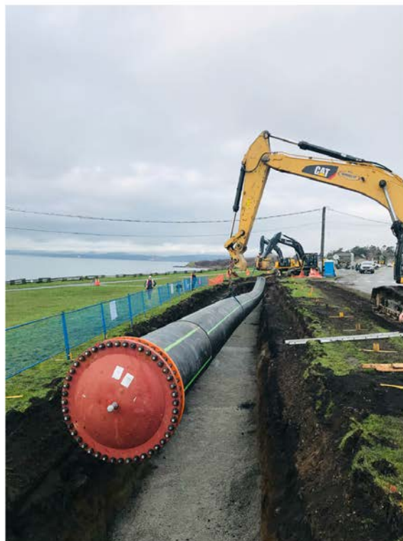
The 1.2m diameter Clover Forcemain is being lowered into the trench near Clover Point. There will be single lane alternating traffic on Dallas Road during construction.
