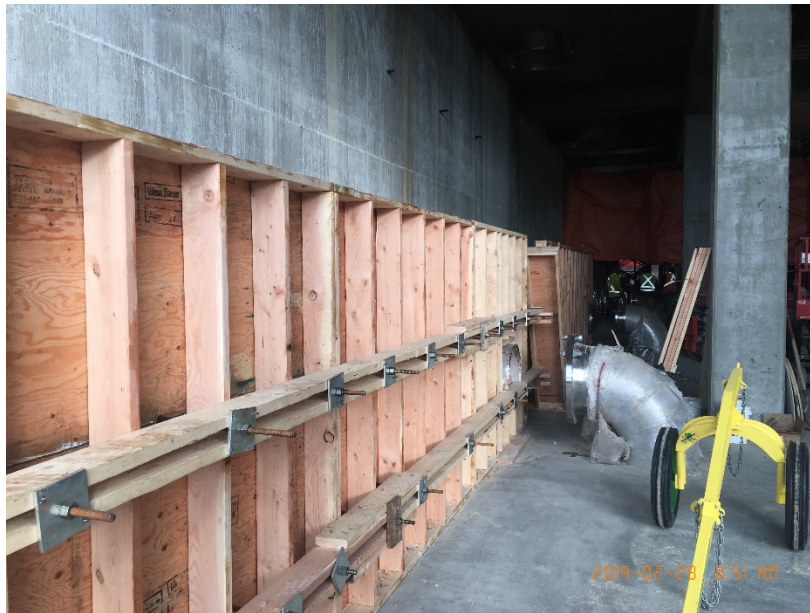
Figure 3 - McLoughlin Point Wastewater Treatment Plant: forming biological aerated filter cell gallery boxes.
