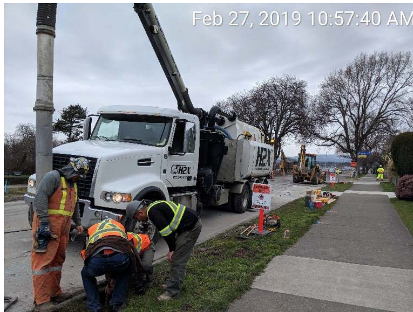
Figure 22 – Clover Forcemain: utility relocates for water between Government Street and Paddon Avenue
