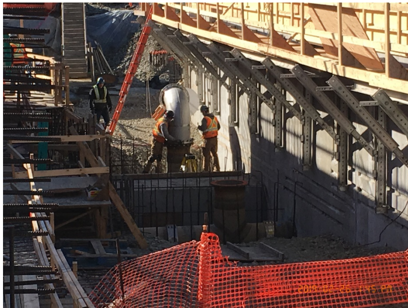
Figure 4 – McLoughlin Point Wastewater Treatment Plant: installing stainless steel risers for moving bed biofilm reactor drains.
