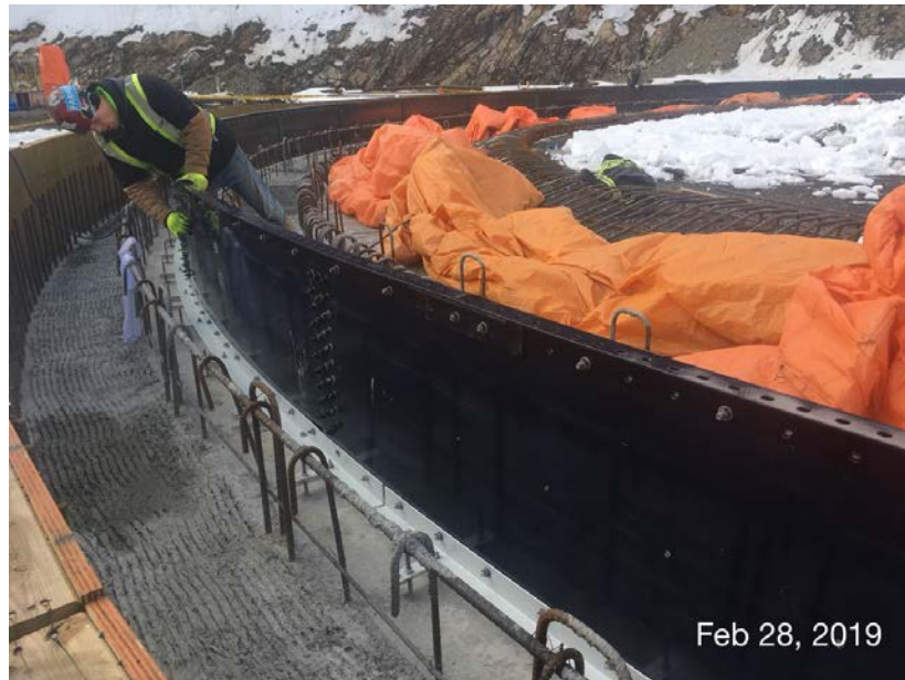
Figure 9 – Residuals Treatment Facility: installation of top angle on bottom row of tank wall plates for digester #1.
