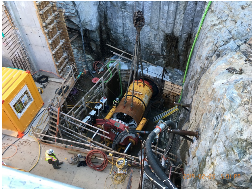
Figure 5 – McLoughlin Point Wastewater Treatment Plant: placing micro tunnel boring machine into launch pit.
