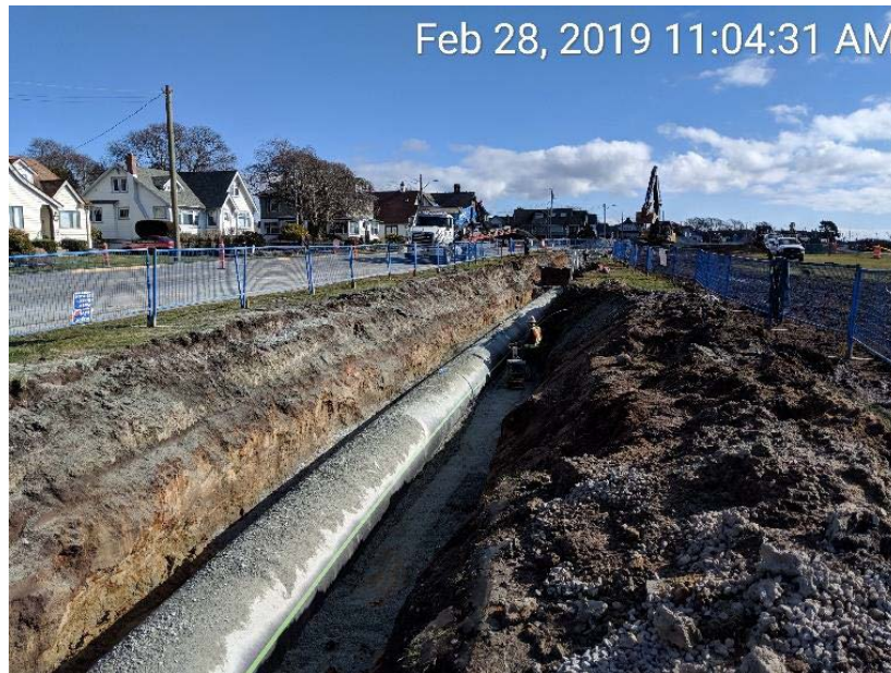
Figure 21 – Clover Forcemain: looking west at backfill and compaction between Marlborough and Cook Streets.
