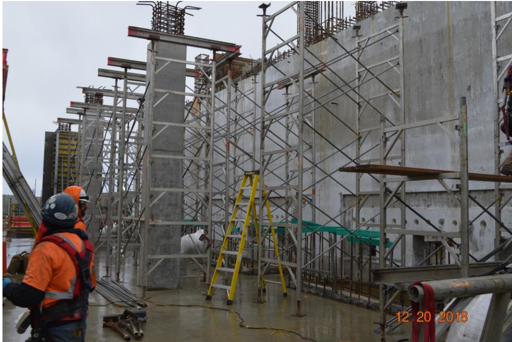
Figure 2 – McLoughlin Point Wastewater Treatment Plant: scaffold erection in biological aerated filter (BAF) gallery for suspended slab formwork.
