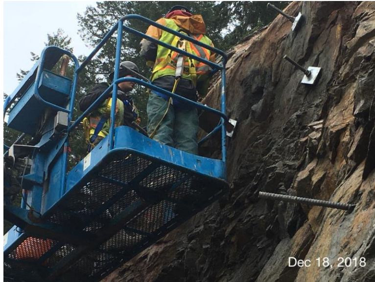
Figure 10 – Residuals Treatment Facility: Testing of rock anchors on south side of digester #2.
