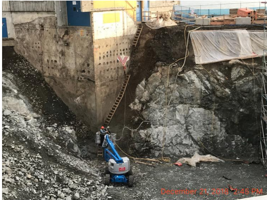
Figure 15 – Macaulay Point Pump Station: Western Grater spraying shotcrete in front of the temporary entrance to the existing facility.
