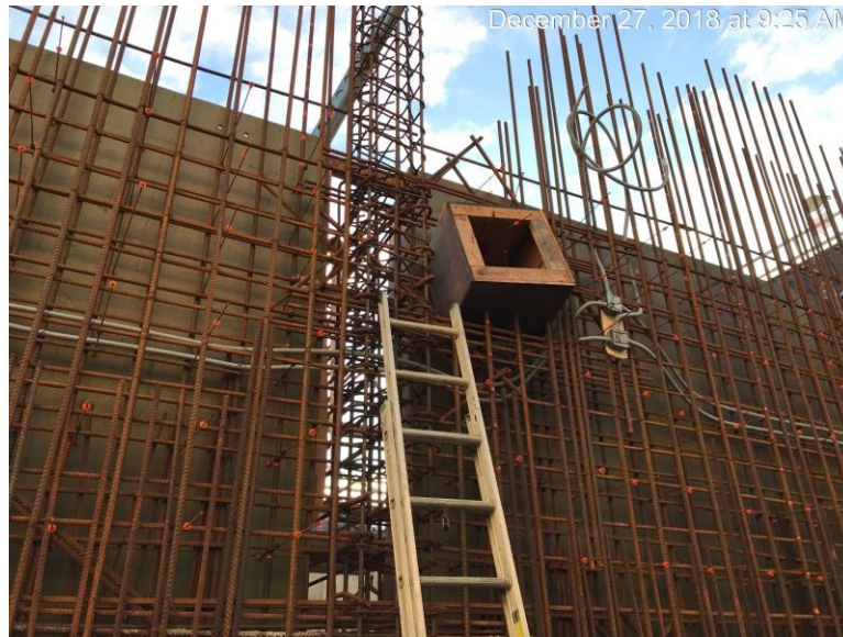
Figure 11 – Clover Point Pump Station: Wall W08 with block out for surge relief drain.
