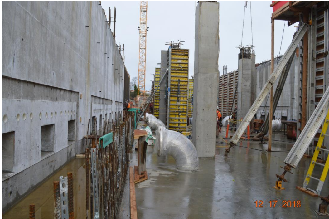
Figure 8 - McLoughlin Point Wastewater Treatment Plant: Biological aerated filter (BAF) pipe gallery looking north.
