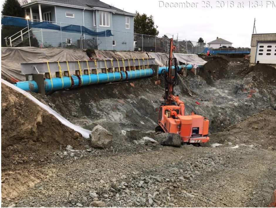
Figure 14 – Macaulay Point Pump Station: Western Grater drilling rock in the south east corner of the site.
