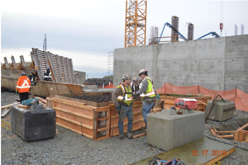
Figure 7 - McLoughlin Point Wastewater Treatment Plant: forming and rebar installation for column foundations at operations and maintenance (O&M) building.
