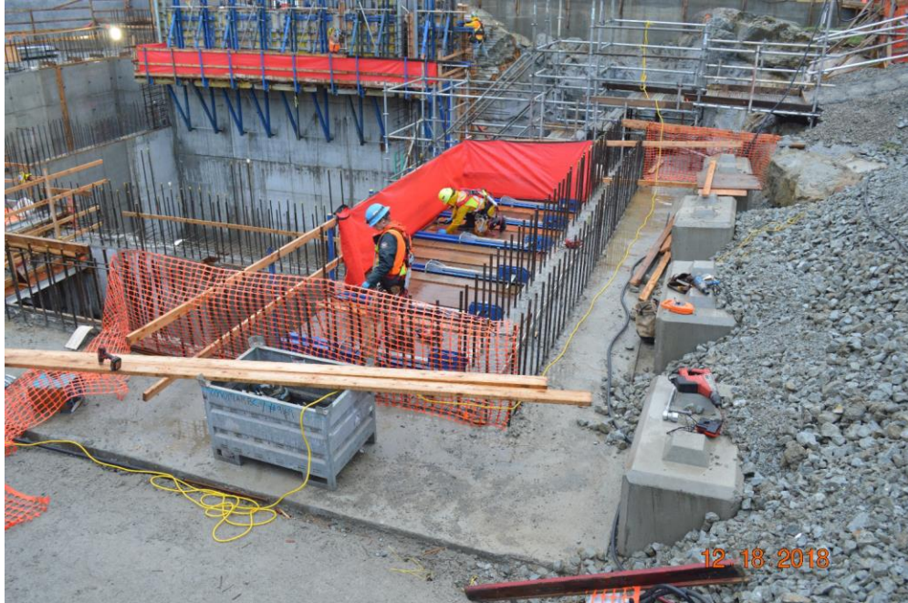
Figure 5 - McLoughlin Point Wastewater Treatment Plant: installing jump deck for wall TB-3-W1 formwork.
