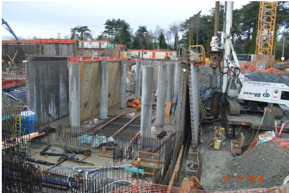
Figure 6 - McLoughlin Point Wastewater Treatment Plant: looking west showing completed columns and walls.
