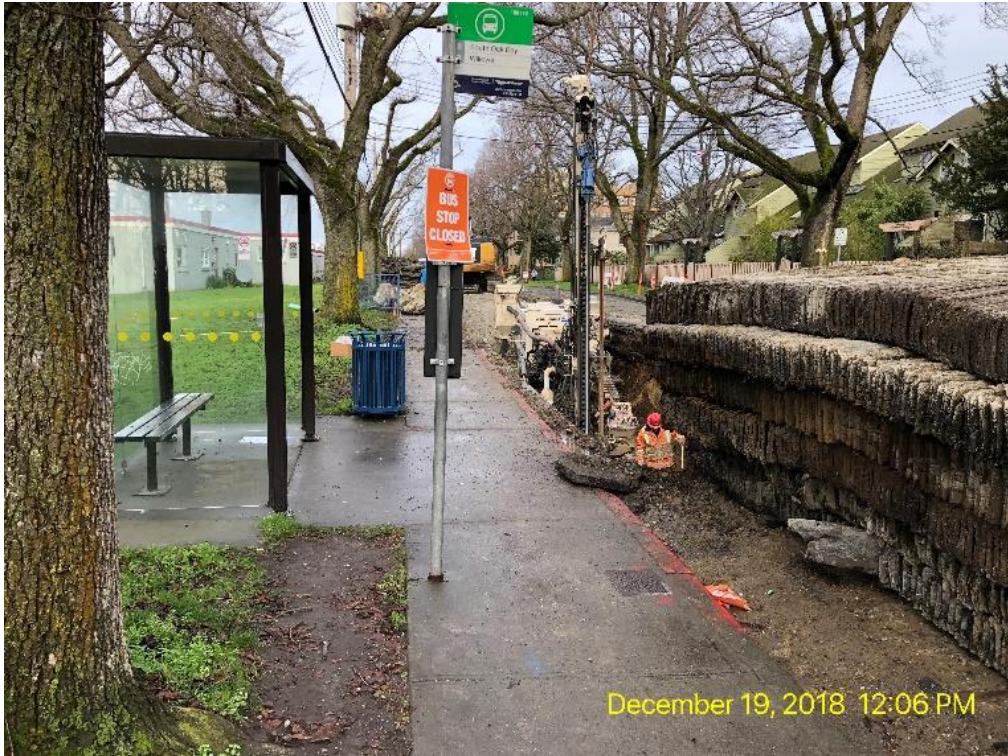
Figure 17 – Clover Forcemain: Dallas Road – Blast mats being placed in preparation for a blast
