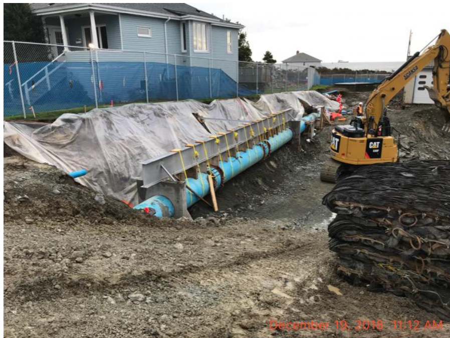
Figure 16 – Macaulay Point Pump Station: looking south at the support of the Western Communities Trunk.
