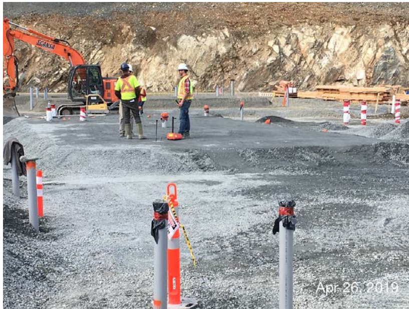
Figure 12 – Residuals Treatment Facility: placing, grading, compaction and shaping of base gravels beneath Residuals Handling Building.
