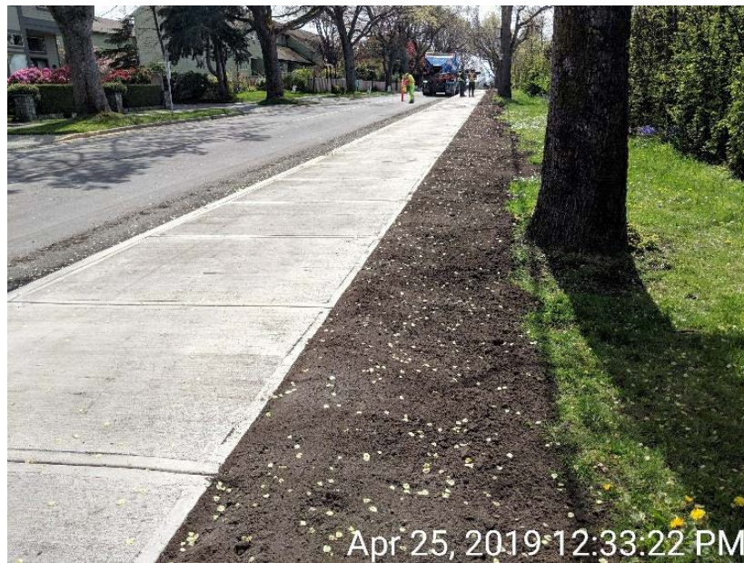
Figure 21 – Clover Forcemain: Dallas Road topsoil placed behind new sidewalk at Ogden Point.
