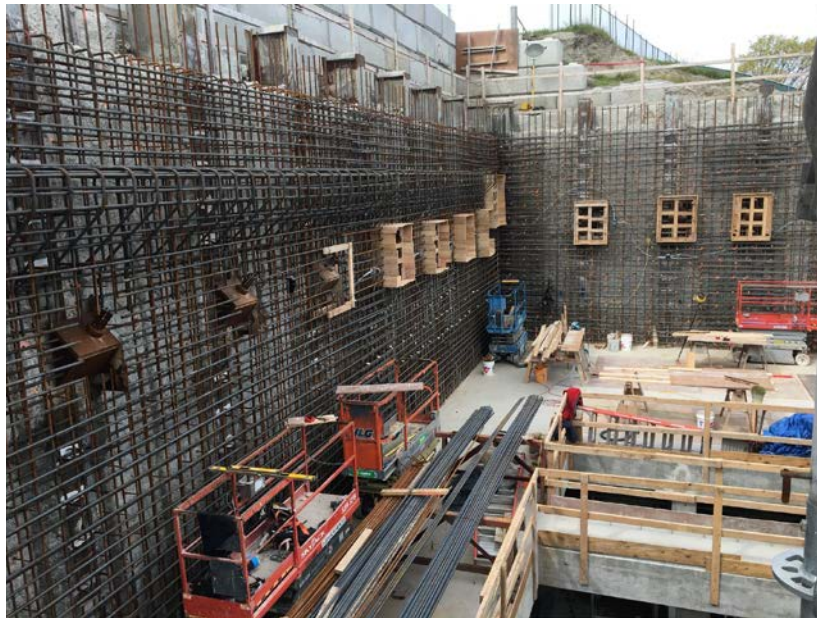
Figure 13 – Clover Point Pump Station rebar, electrical and block outs for wall 33A and 35A.
