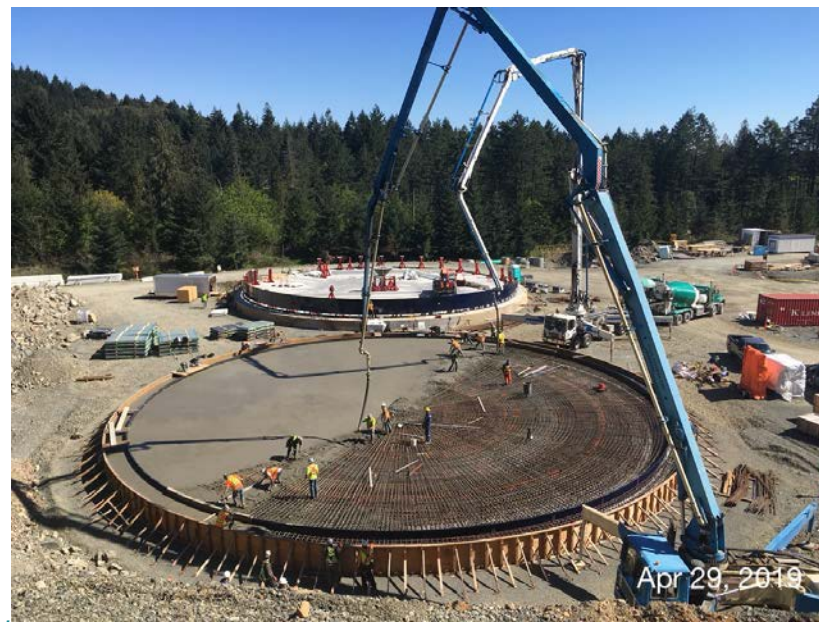
Figure 11 – Residuals Treatment Facility: concrete being placed in digester #2 floor slab and erection of bolted steel tank wall in the background.
