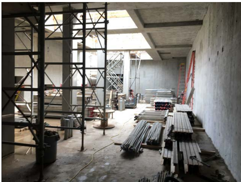
Figure 14 – Clover Point Pump Station: pump room (view from south).
