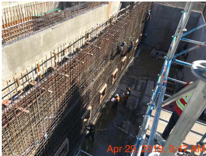
Figure 19 – Macaulay Point Pump Station: installing rebar, electrical conduits and formwork for interior wall along gridline C.
