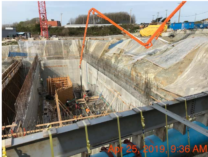
Figure 20 – Macaulay Point Pump Station: concrete pour of the topping slab in the inlet channel.
