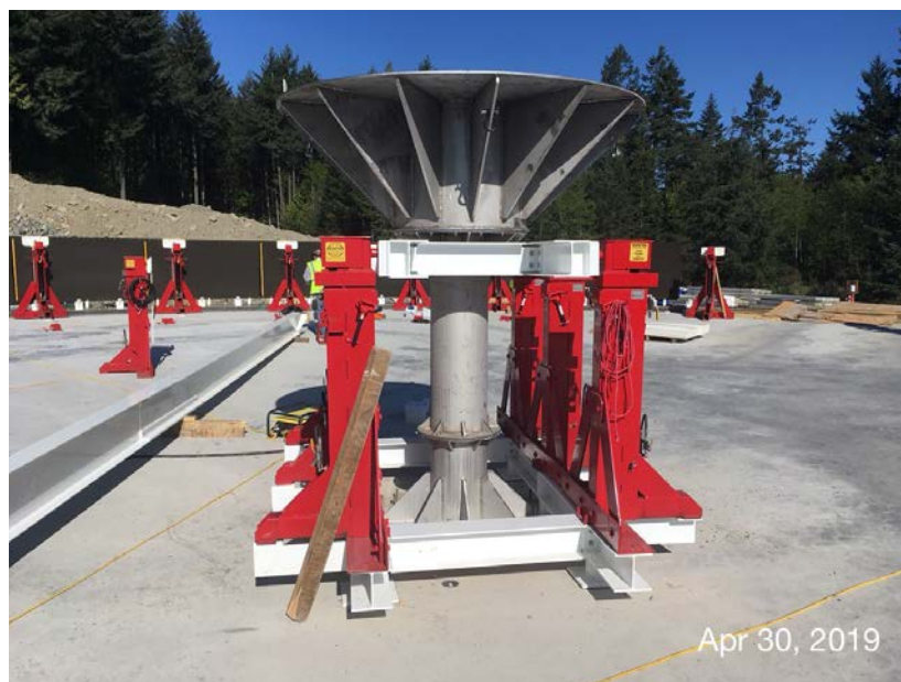
Figure 9 – Residuals Treatment Facility: hydraulic jacks set up around central roof support column.
