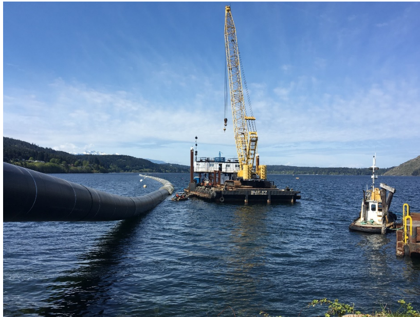
Figure 3 - McLoughlin Point Wastewater Treatment Plant: Assembly of marine outfall pipe in Nanoose Bay.
