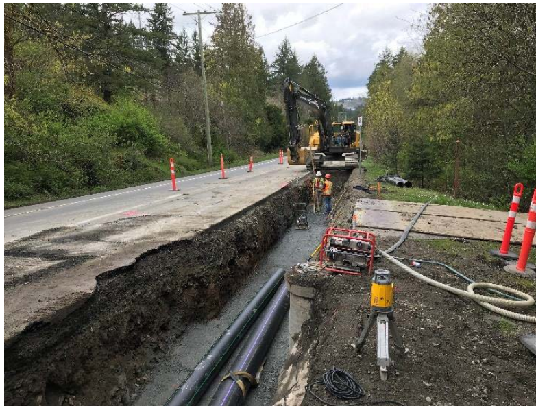
Figure 25 – RSCL: Segment 3 - installation of residual solids forcemain and centrate return line at Interurban Road.
