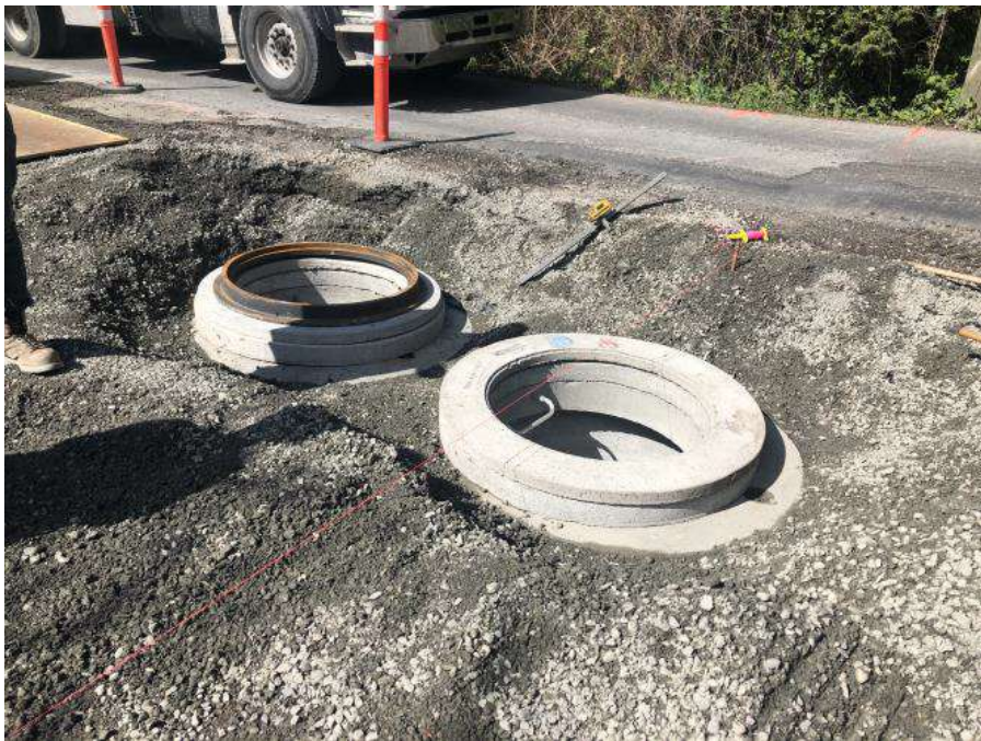
Figure 19- Residual Solids Pipes- Setting of grade rings at low point drain on Interurban Road.
