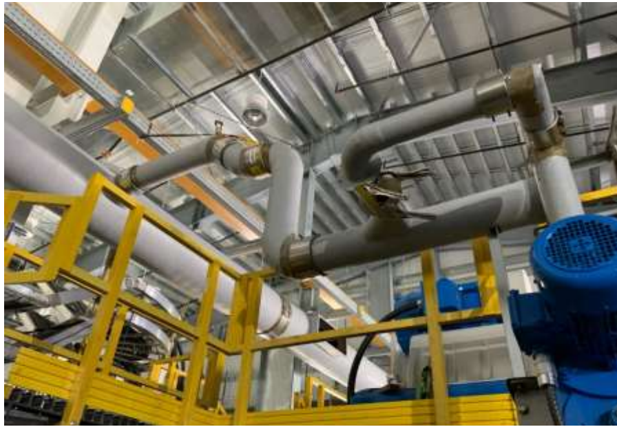
Figure 9– Residuals Treatment Facility- Installation of fibreglass ducting for odour control system ongoing in Residuals Handling Building.
