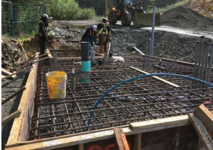
Figure 23 –Residual Solids Pump Stations – Pump Station 3 Installing formwork and rebar for odour control unit slab.
