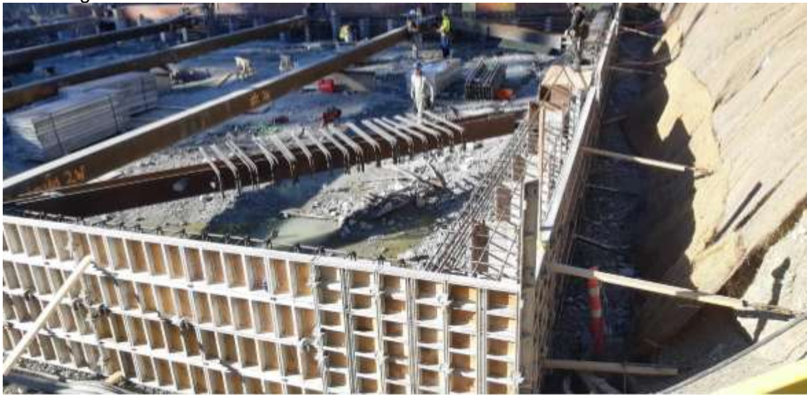
Figure 24–Arbutus Attenuation Tank–Installed diagonal and lateral struts atop the secant piles, formwork and rebar installed for section 1 of ring beam.
