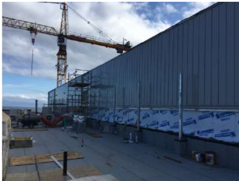
Figure 6- McLoughlin Point Wastewater Treatment Plant- Installing aluminium cladding on east face of Heat Recovery Room.
