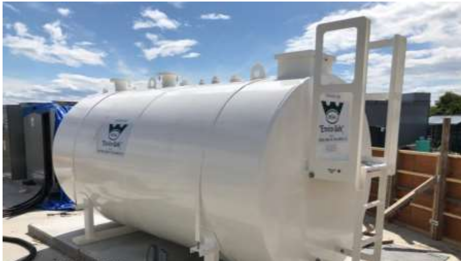
Figure 15–Macaulay Point Pump Station- Fuel tank positioned in containment area.
