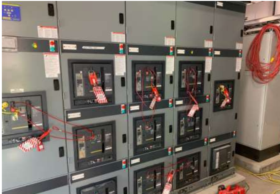
Figure 7– Residuals Treatment Facility- Wiring of Residuals Handling Building Motor Control Centre/electrical room nearing completion.
