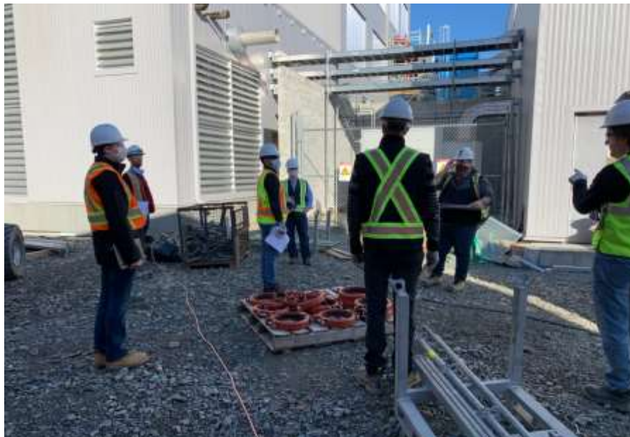
Figure 8– Residuals Treatment Facility- Main power distribution –Construction walk down and punch list preparation being undertaken.
