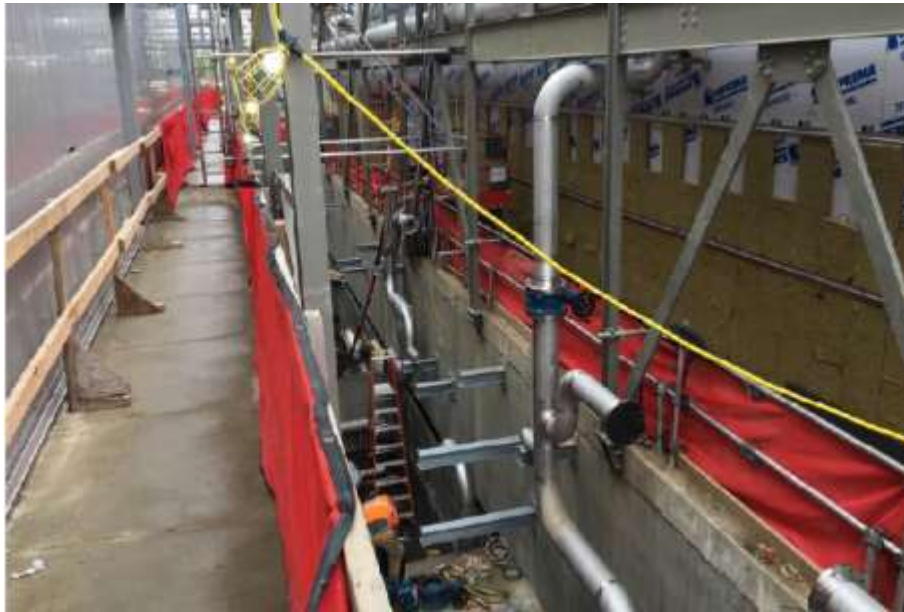
Figure 5- McLoughlin Point Wastewater Treatment Plant- Installing process air piping to Biological Aerated Filter cells 2, 4, 6, 8, 10, and 11.
