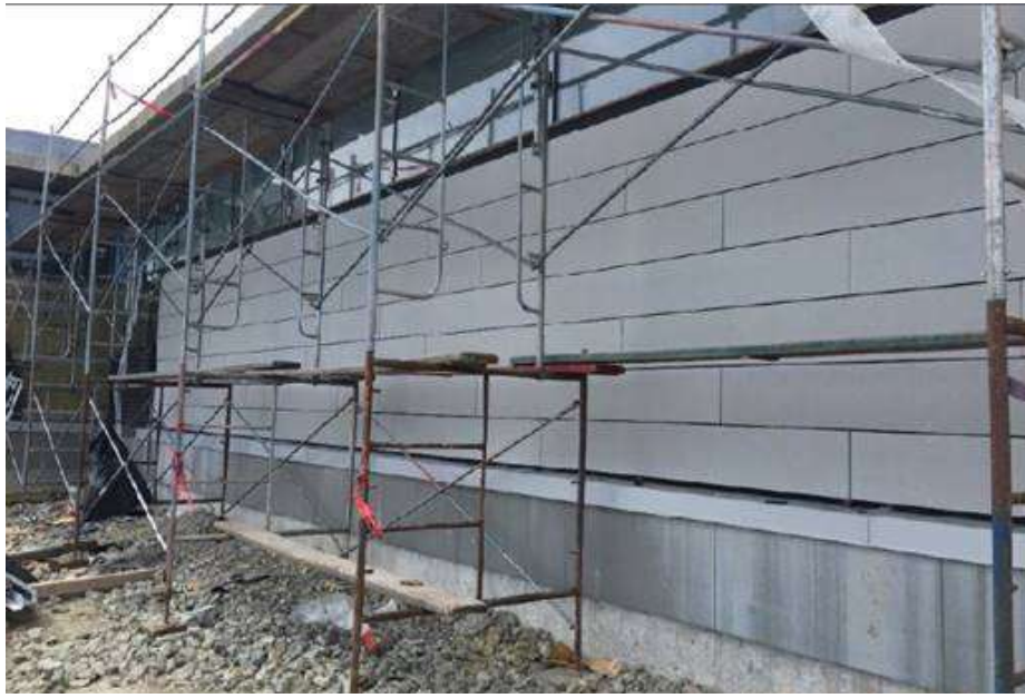
Figure 3– McLoughlin Point Wastewater Treatment Plant- Installing concrete architectural panel on operations and maintenance building.
