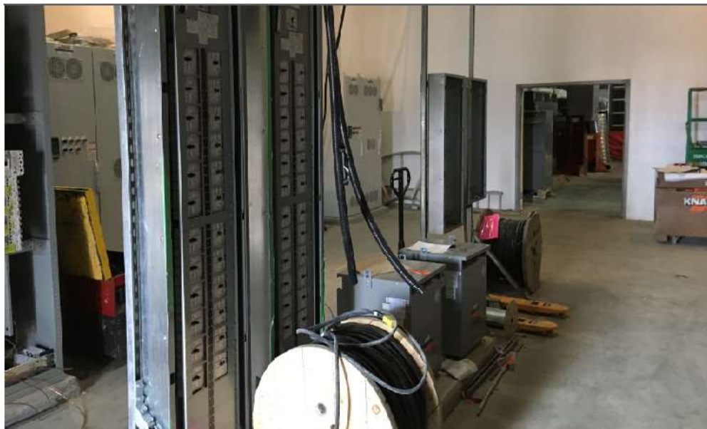
Figure 4– McLoughlin Point Wastewater Treatment Plant- Installing distribution and lighting panel boards in blower electrical room.
