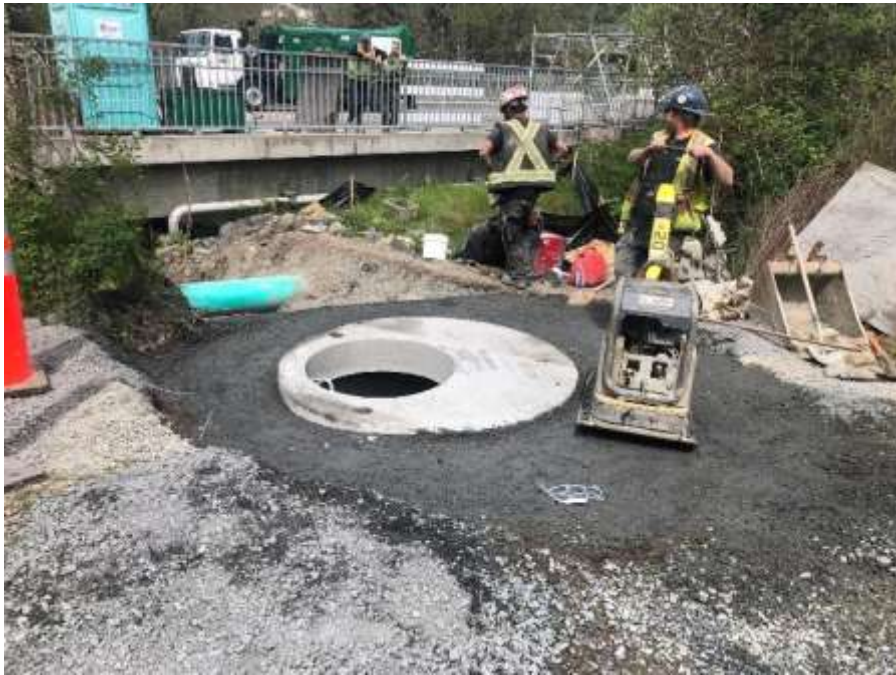
Figure 18- Residual Solids Pipes- Backfill and compaction around line valve at Admirals Bridge.
