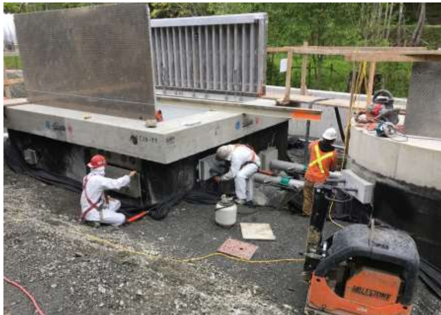
Figure 22–Residual Solids Pump Stations– Pump Station 1 – Grouting and sealing of pipe penetrations in valve chamber.
