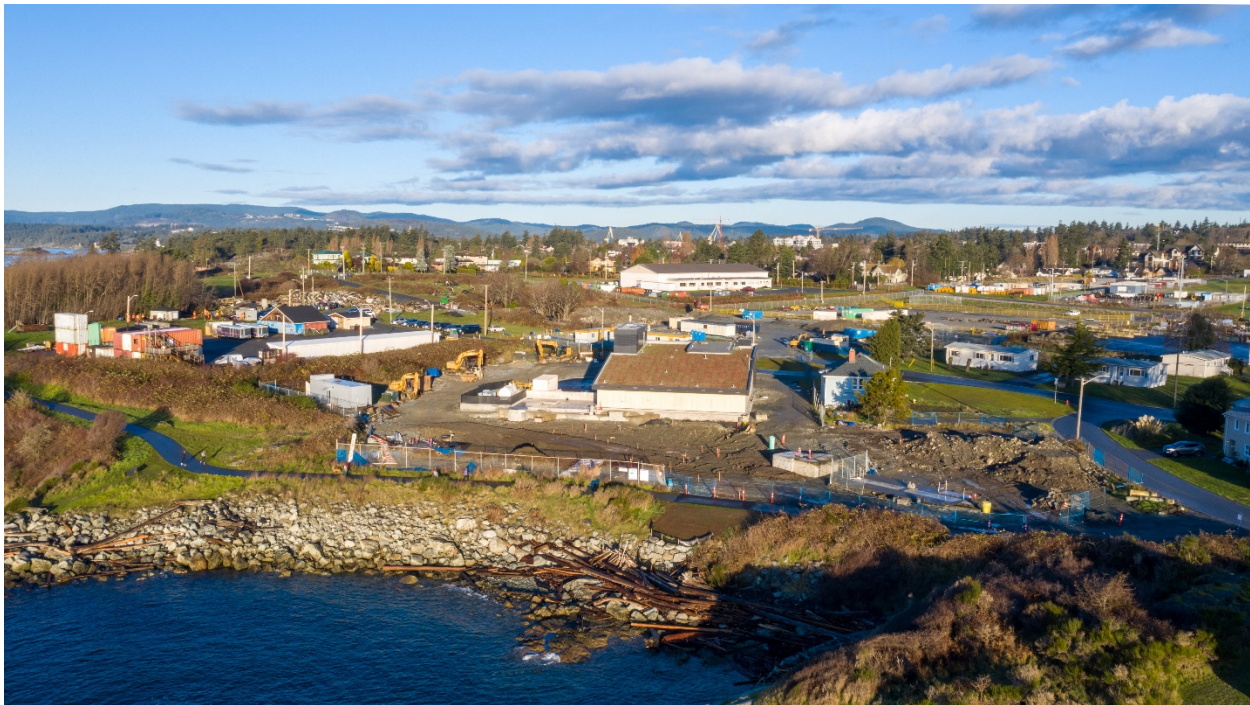
Figure 10 – Looking north towards the Macaulay Point Pump Station (construction in progress, landscaping still to be completed)
