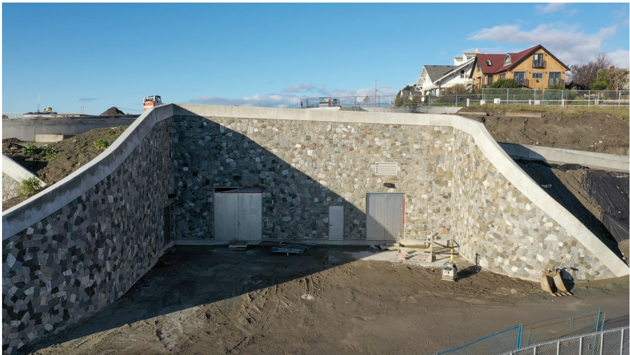
Figure 6 – Entrance to the expanded Clover Point Pump Station (construction in progress: public amenities and landscaping still to be completed)
