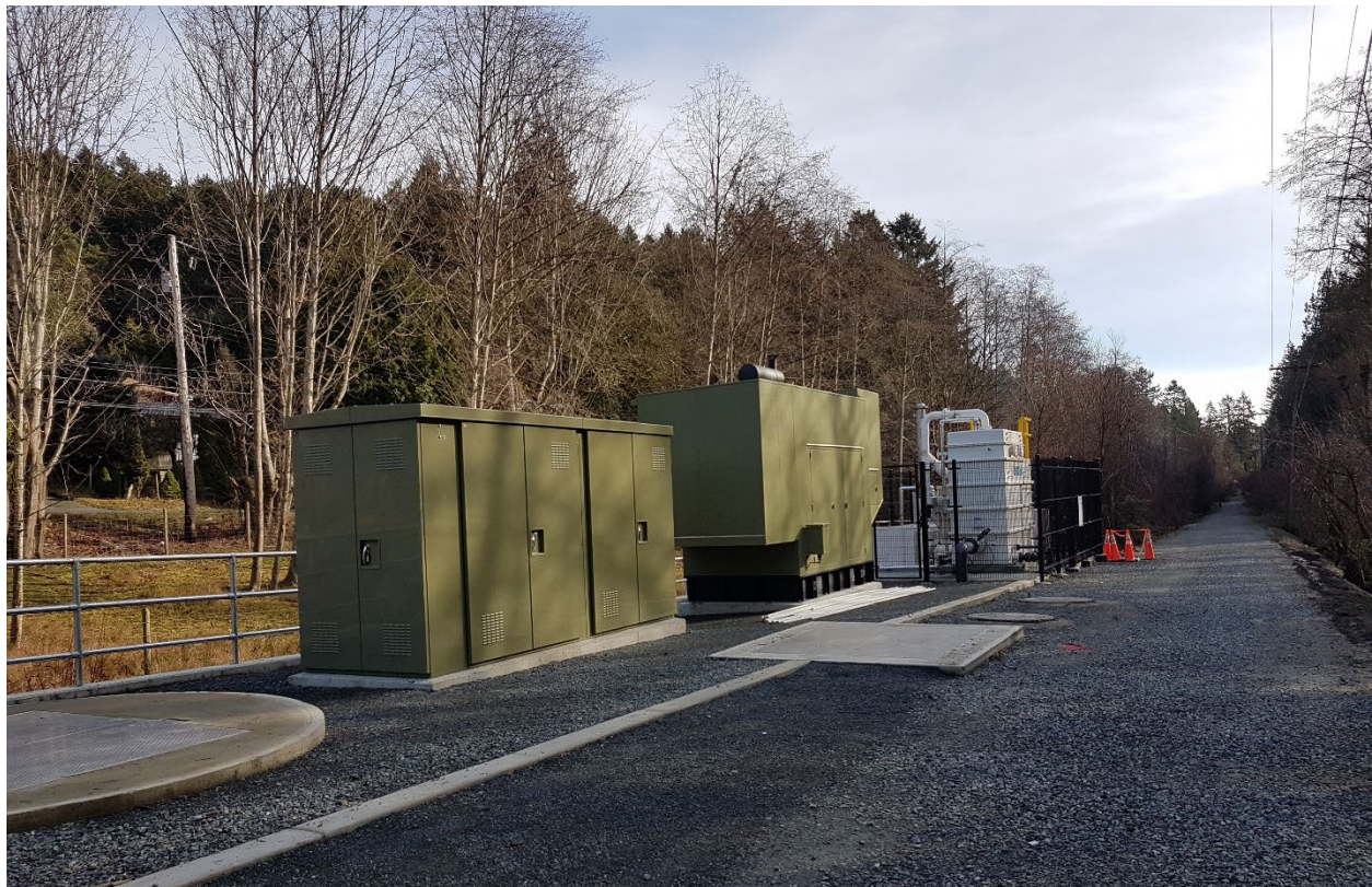
Figure 12 – Residual Solids Pump Station located along the Interurban Rail Trail in Saanich (Construction in progress, landscaping still to be completed)
