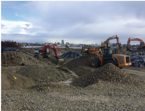
Excavation at McLoughlin Point is underway as crews prepare the site for the construction of the new McLoughlin Point Wastewater Treatment Plant.
