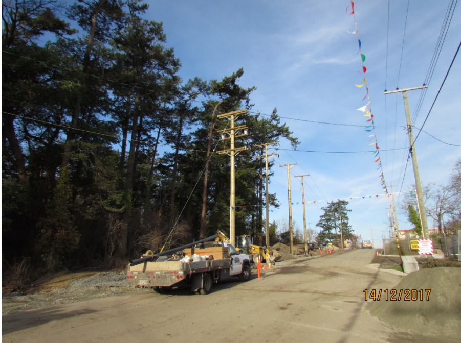
Figure 4 – New BC Hydro power poles and lines on Victoria View Road
