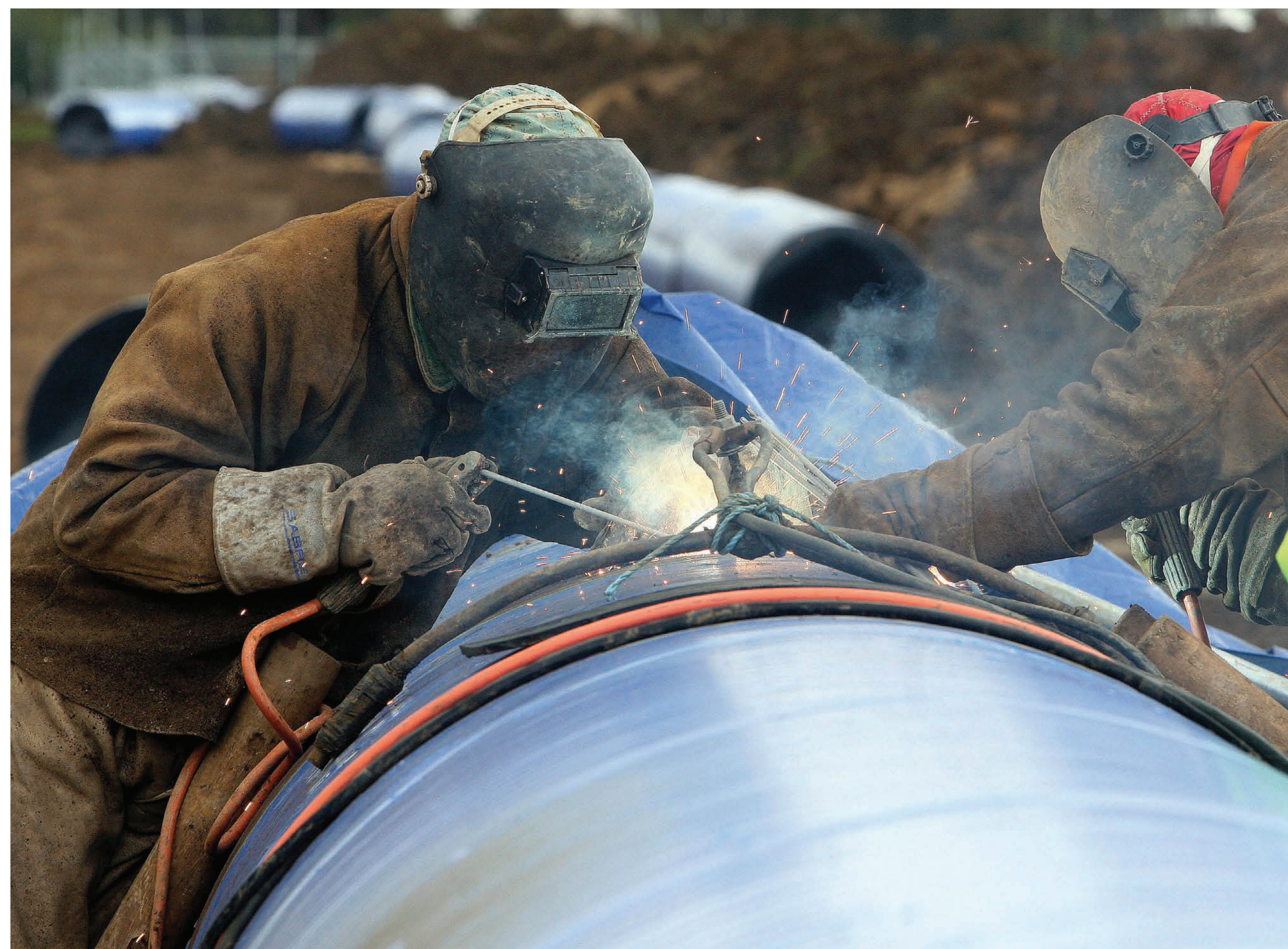
Welding of the sections of pipe will take place within an enclosure
