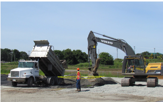
Crews placing aggregate in a laydown area for the McLoughlin Point Wastewater Treatment Plant in Esquimalt.
