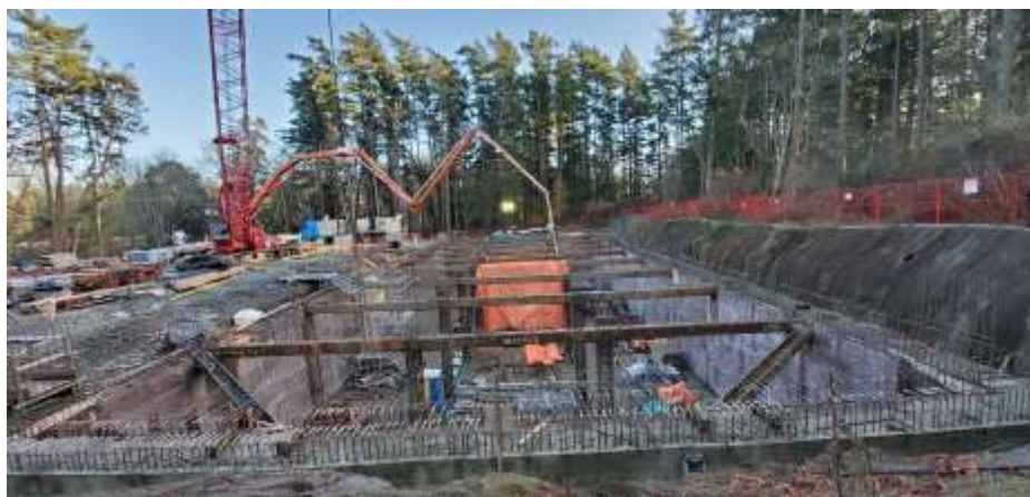
Figure 13 – Arbutus Attenuation Tank- Attenuation Tank Overview.
