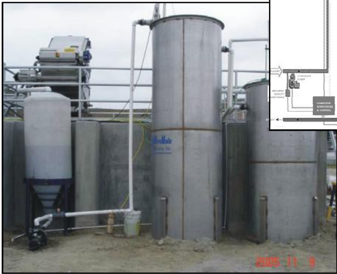
Complete CleanStream™ system: sludge separator, equalization tank, and CBUM filtration columns.
