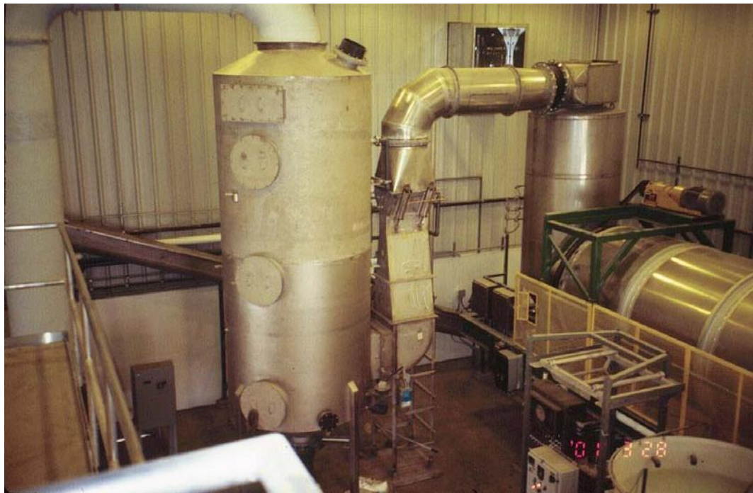
CONDENSOR/SEPARATOR, VENTURI SCRUBBER, CYCLONE SEPARATOR
