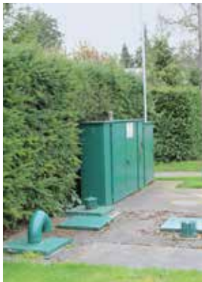
>> Uganda Ave. Pump Station
