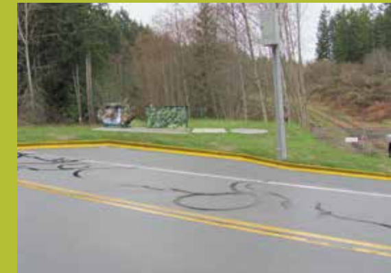
>> Willis Point Road Pump Station
