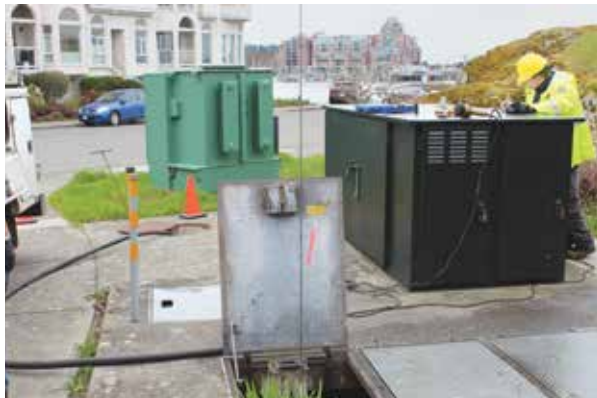
>> Cooperage Place Pump Station (above and right)
