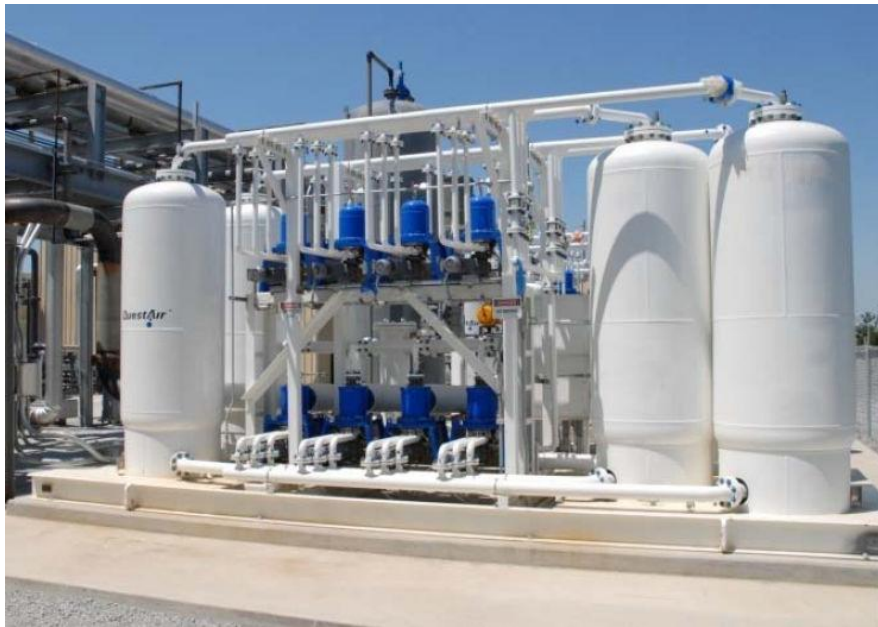
Figure 6.3 – QuestAir PSA System at Rumpke Landfill, Ohio
