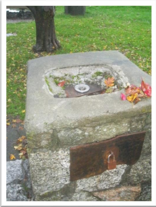
Photo 17: Water fountain in disrepair. It should be fixed because every good park deserves a good water fountain.
