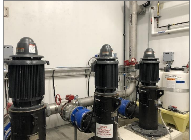
Figure 1-1 NSSWD St. Mary Lake Treatment Plant pumps
