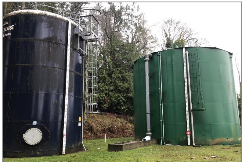
Figure 1-2 NSSWD Storage Tanks
