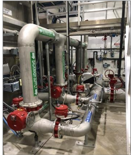
Figure 1-NSSWD St. Mary Lake Treatment Plant piping
