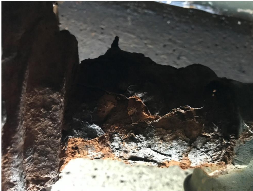
Photograph #5 – Bottom View: 50 mm dia. Irrigation Feed Deposit build up and suspect spalling
