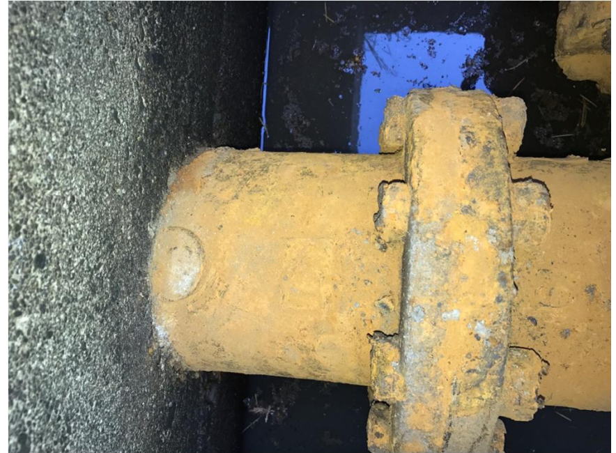
Photograph #8 – Top view: 150 mm Upstream flanges and hardware at concrete chamber wall interface
