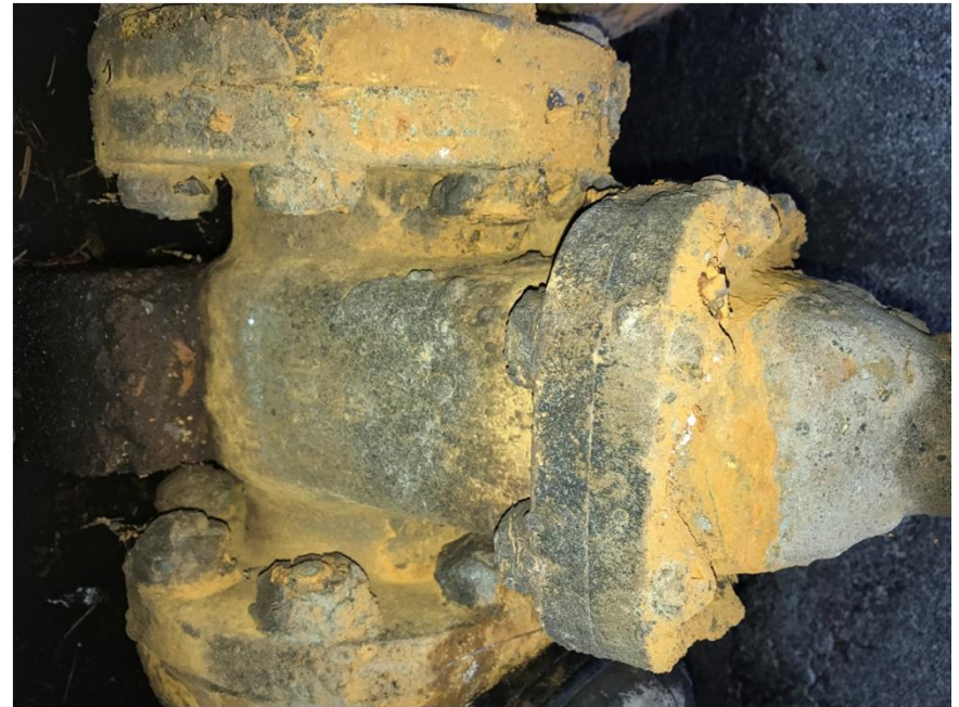
Photograph #10 – Side View: 150 mm Low Level Outlet Control Valve, flanges, nuts & bolts
