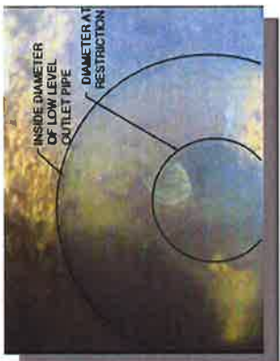
PHOTO 1 (PIPE RESTRICTION - FROM PIPE VIDEO INSPECTION, JAN 13, 2015)
