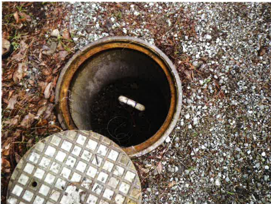
Photo 10: Valve cover for nearby well (Feb. 13, 2013).
