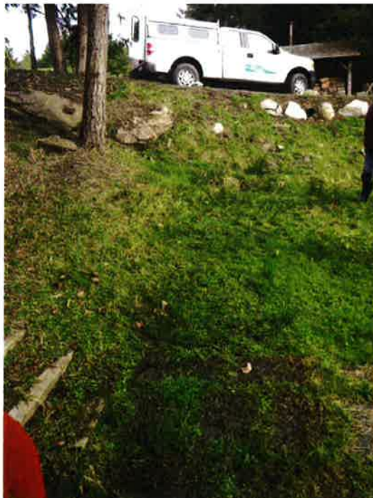
Photo 6: Seepage area downstream of dam (Feb. 13, 2013).
