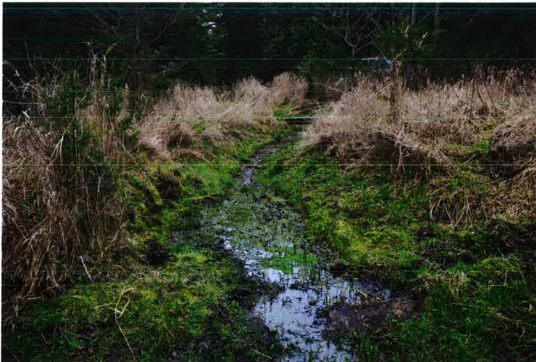
Photograph #6 – Existing Spillway Channel looking Downstream towards Gardom Lane (from Photo #5 location)
