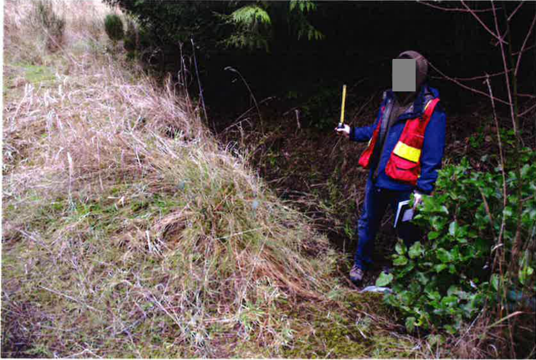
Photograph #7 – Existing Spillway Cross Section from Pond to Approx. Location of Photo #5
