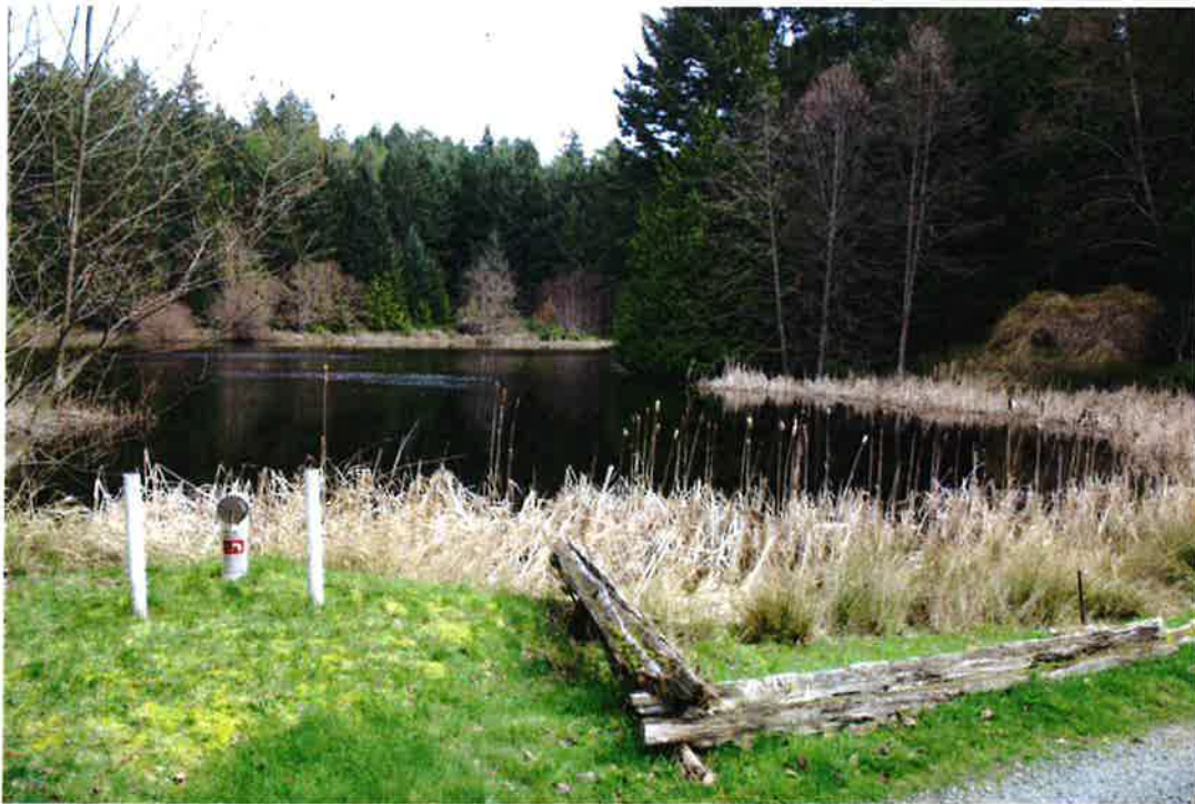
Photograph #8 – Location of RPID Emergency Fire Supply Standpipe
