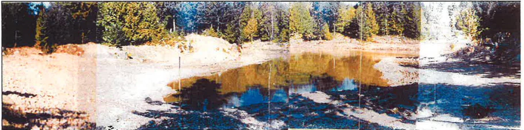
Panorama Cross, Downstream Face of Dam and Reservoir from Left Abutment - March 20, 1979
