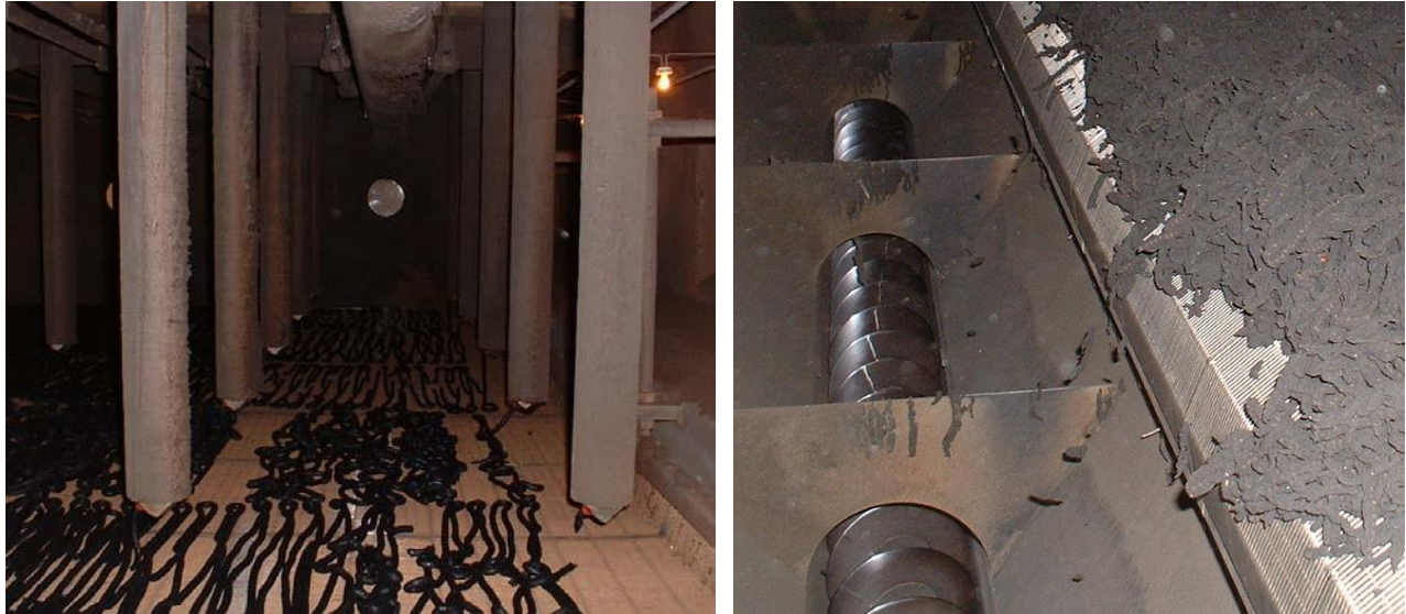
Figure 5.7 – Inside the Belt Dryer, Randers, Denmark
