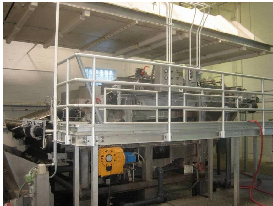
Figure 5.1 – Andritz Belt Filter Press: Salmon Creek WWTP, Vancouver, Washington
