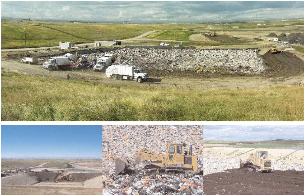
Figure 3.13 – Biocell in Operation (Stantec, 2006)
