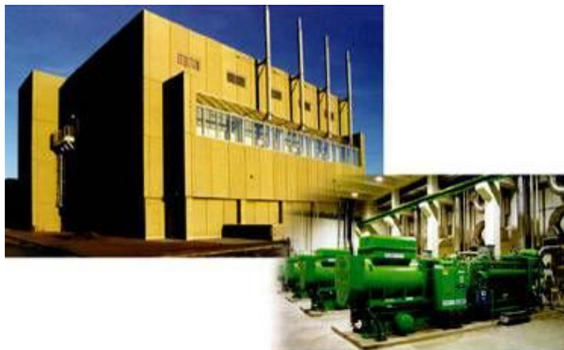
Figure 6.2 – 4-MW Cogeneration System at Metro Vancouver’s Annacis Island WWTP
